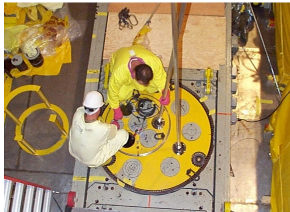
Figure 3-19. Example of a rotating-plug maintenance shield used at ORNL.
