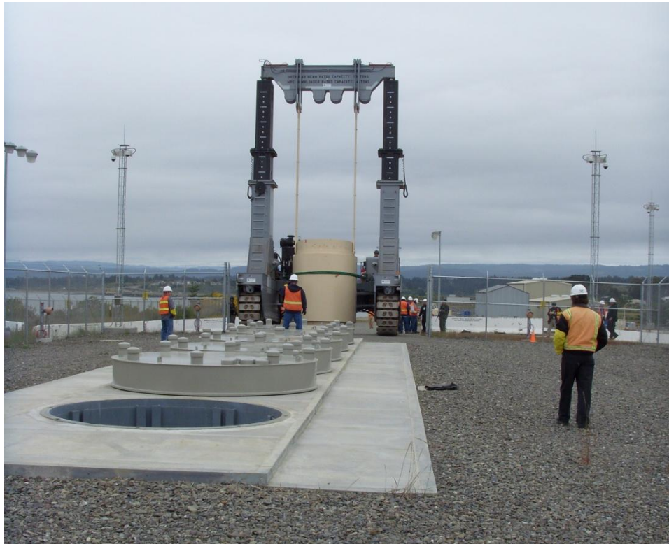
Figure 2-6. Humboldt Bay Underground HI-STAR Independent Spent Fuel Storage Installation (Photo courtesy of Holtec International; reprinted with permission)
