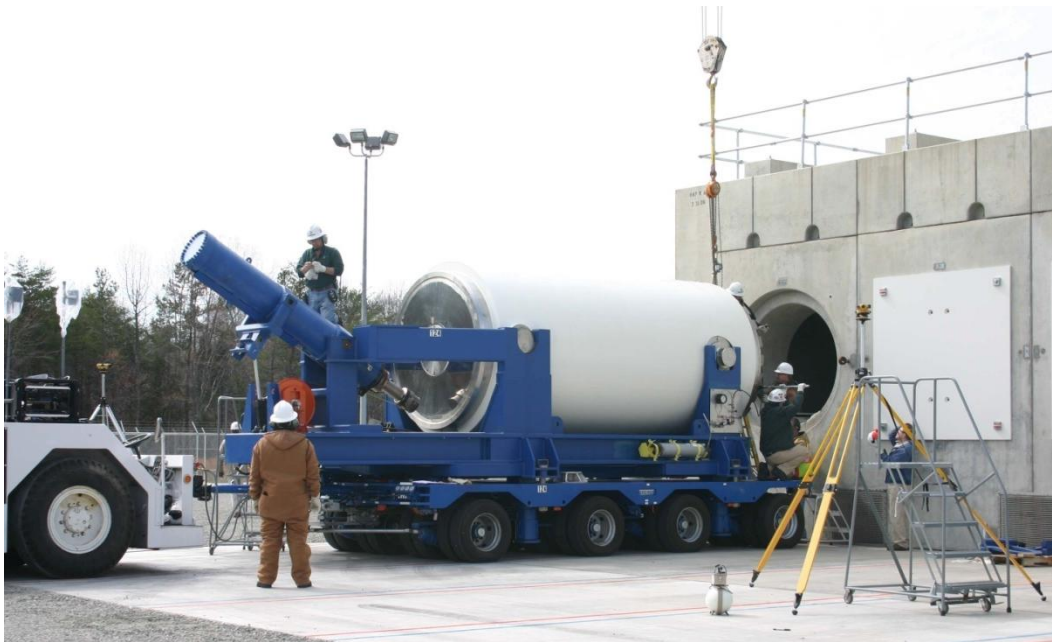
Figure 2-8. NUHOMS Dry Storage Cask Being Loaded into the Horizontal Storage Module (Photo courtesy of Transnuclear, Inc.; reproduced with permission)
