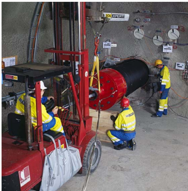
Figure 3-26. HG-A Experiment at Mont Terri URL: Installation of packer system (from Marschall et al., 2012).
