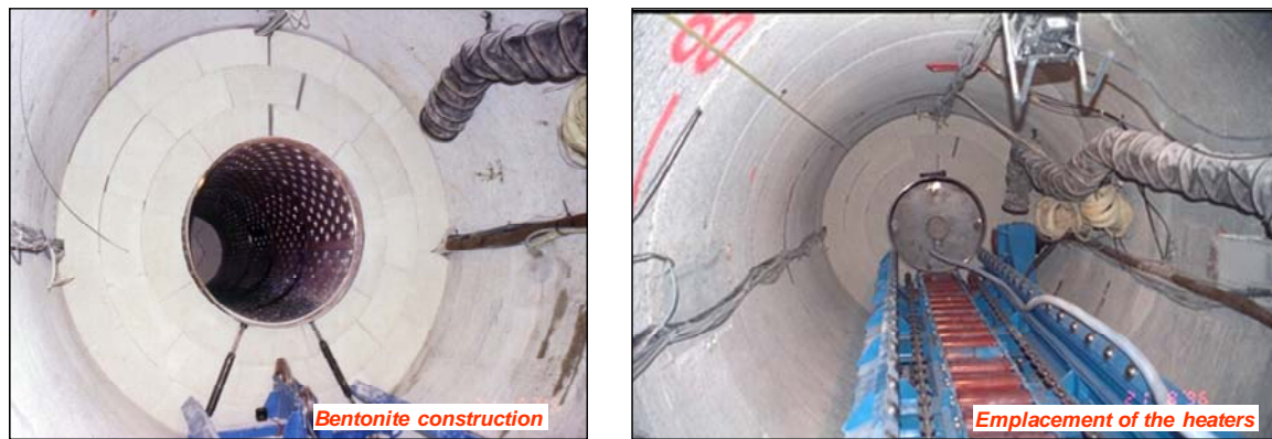
Figure 4-8. FEBEX Test at Grimsel Test Site: Photos taken during the construction phase of the FEBEX test.
