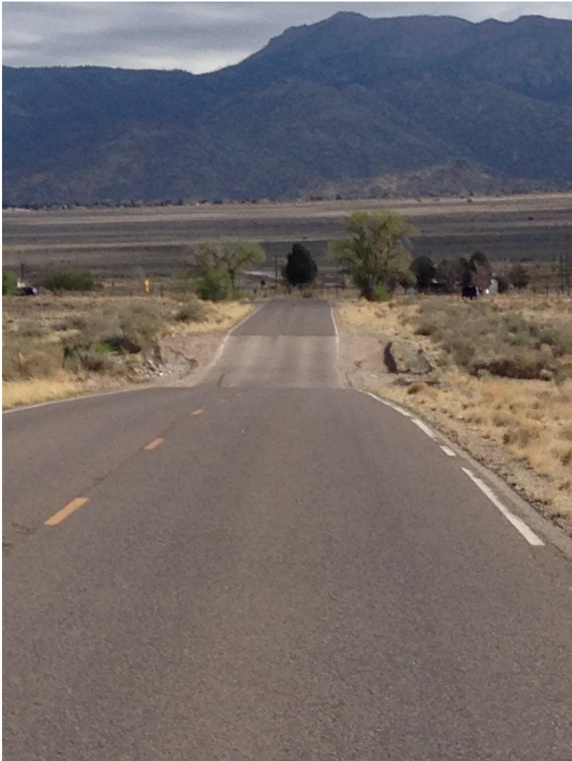
Figure 4.6 Dip on Area III road approaching Pennsylvania St., Segment 1 (going north near beginning of truck route) and Segment 5 (going south near end of test).
