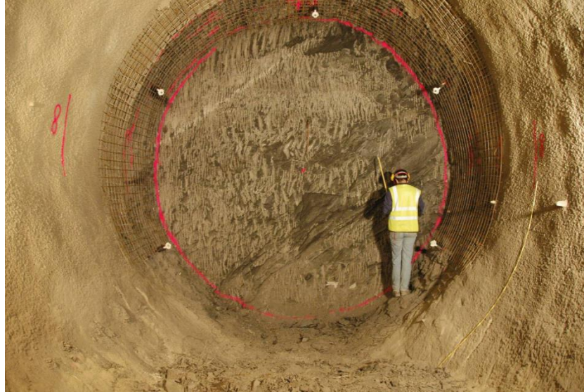
Figure 4-24. View of FE tunnel face from the FE niche showing beddings dipping 45^\circ (Vietor, 2012).
