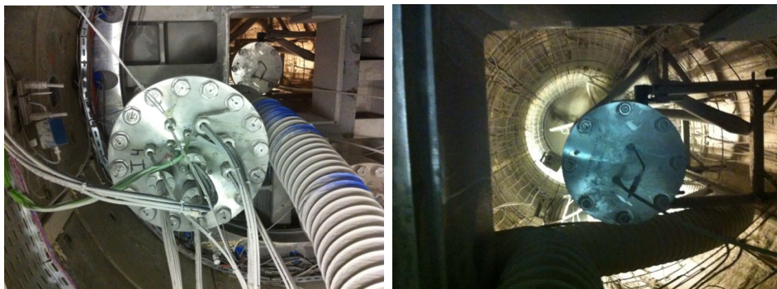
Figure 4.5-4 PRACLAY in situ experiment at HADES URL: Photo on left shows hydraulic seal from the outside, with an access hole to the right, which soon will be closed. Photo on right was taken from access hole into the heater gallery section, which is currently being backfilled.
