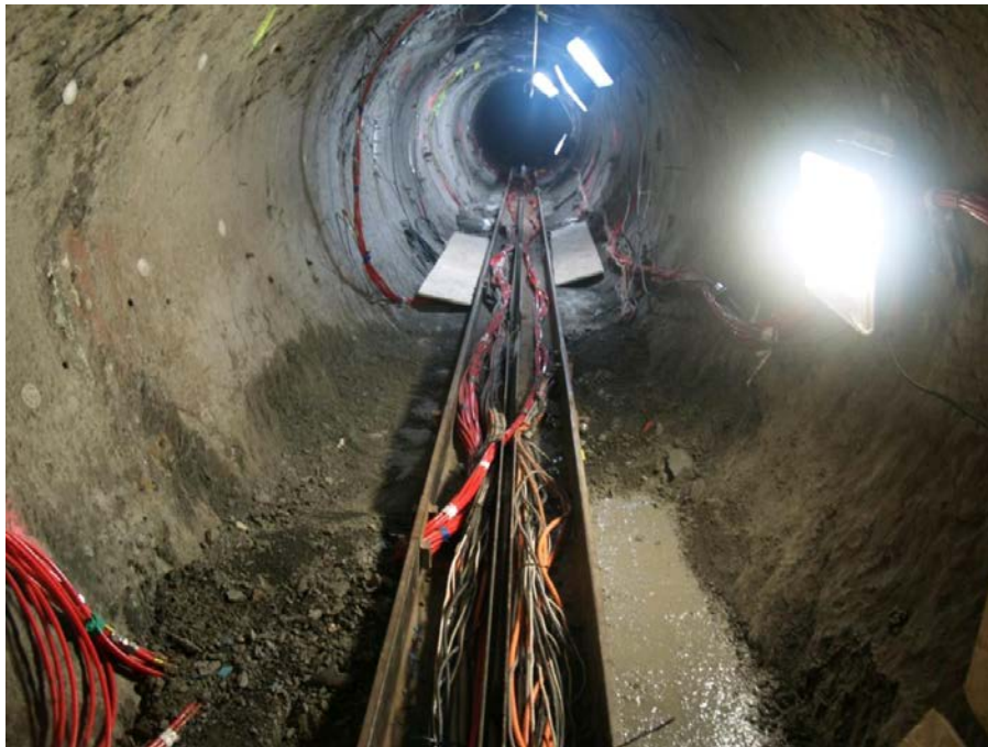
Figure 3.1-10 HE-E Heater Test at Mont Terri URL: Photo of micro-tunnel before buffer emplacement.
