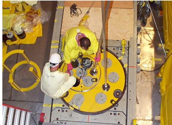
Figure 3-17. Example of a rotating-plug maintenance shield used at ORNL.
