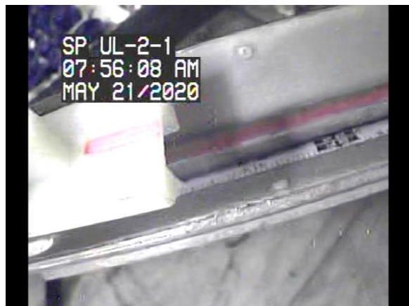
(a) Orange Lateral Mark on Segment UL-2
