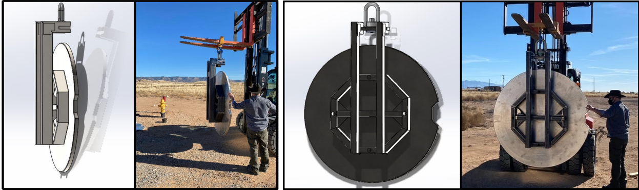
Figure 2.2 Lid lifting fixture allows lid to be installed into canister horizontally.
