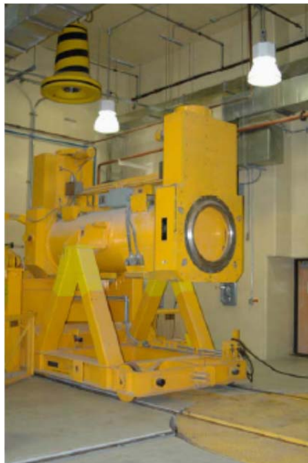
Figure 5-22 A Facility Cask Is Moved Into The Unloading Station And Rotated To A Vertical Position To Receive The Waste Canister
