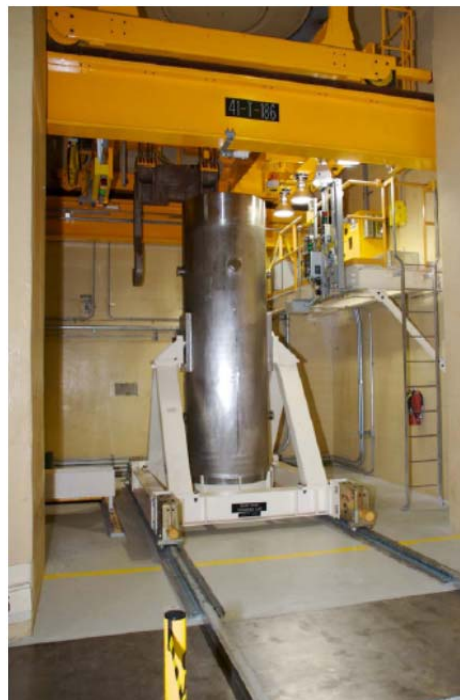
Figure 5-20 A Transportation Cask Is Moved By The Transfer Car Into The Cask Unloading Room
