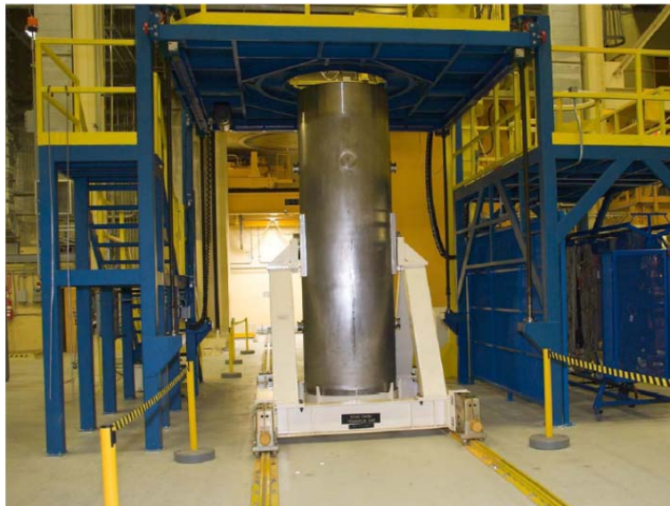
Figure 5-18 A Transportation Cask Loaded On a Cask Transfer Car At The WHB Receipt Bay Inspection Station
