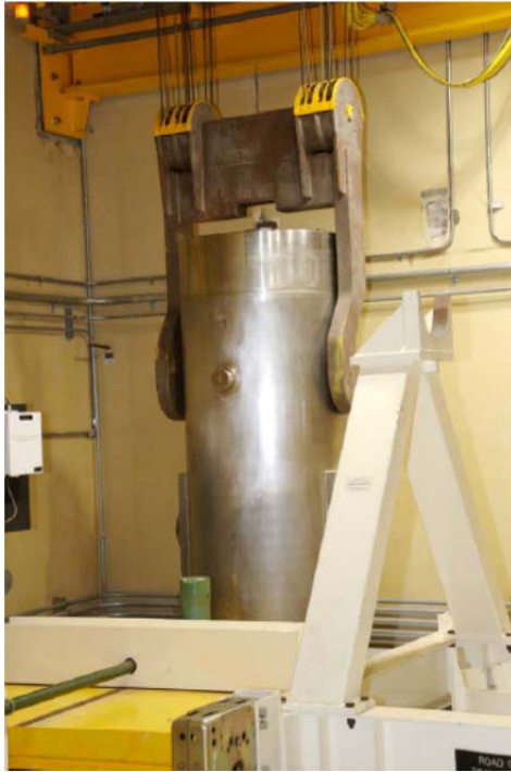
Figure 5-21 A Transportation Cask Is Lowered Into The Transfer Cell
