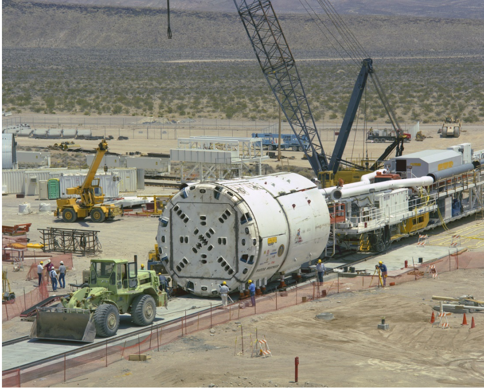
Figure 1. Open-type double-shield TBM with trailing gear, during assembly, Yucca Mountain, Nevada (diameter 7.6 m).
