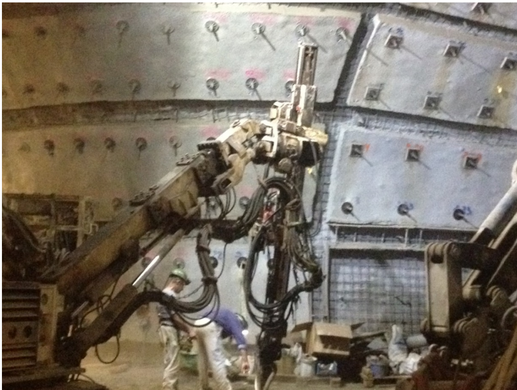
Figure 8. Yielding initial support (wire fabric, shotcrete and long rock bolts) just after installation in the Lower Cretaceous clay at the Konrad repository site (depth ~1,000 m; photo by author).
