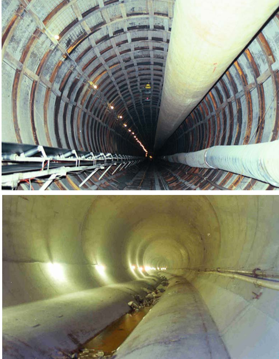
Figure 9. Mill Creek Tunnel Phase 2 (Cleveland, OH) showing steel ribs and lagging support (upper) and final cast-in-place concrete liner (lower) (with permission, HMM 2010).
