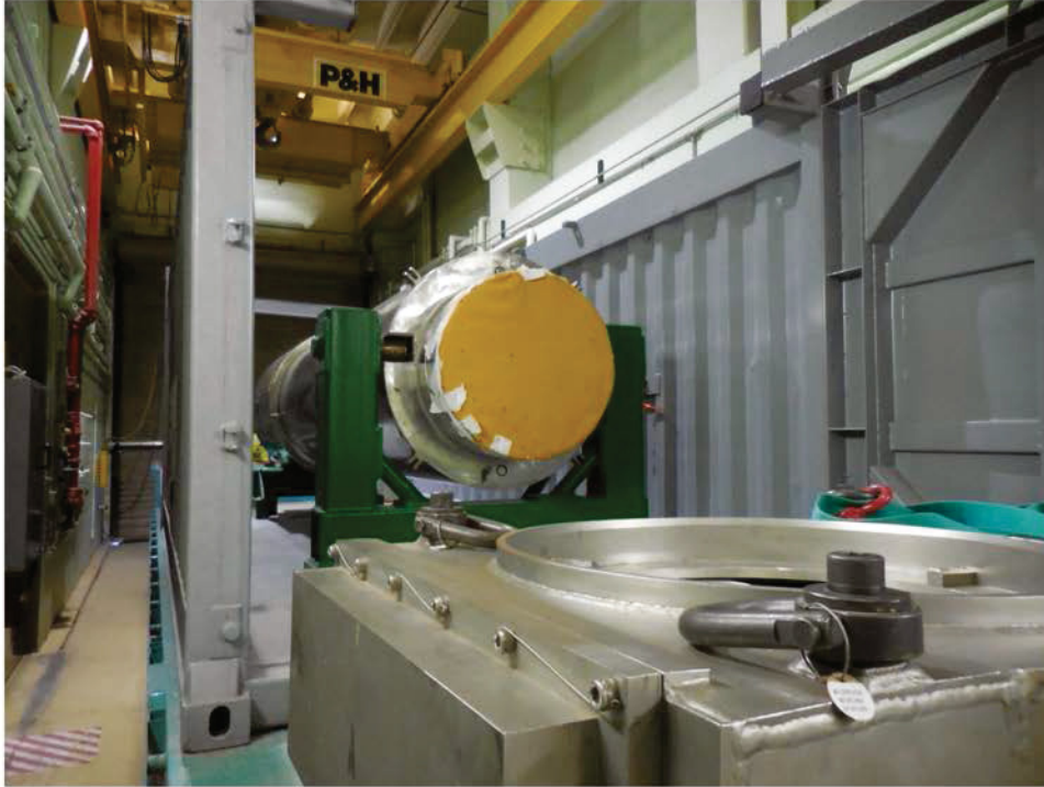
Figure 1. NAC-LWT cask in background with NAC-provided shutter shield in foreground during dry run operations at HFEF.
