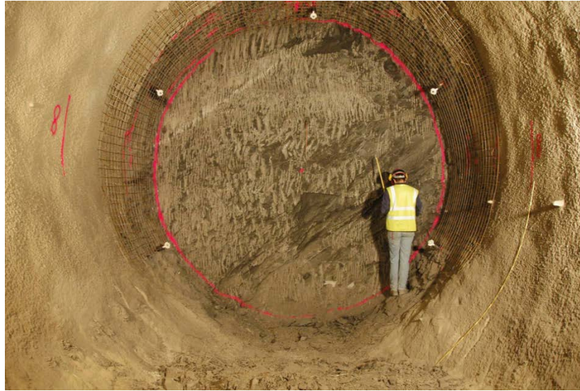
Figure 4.38. View of FE tunnel face from the FE niche showing beddings dipping 45° (Vietor, 2012).
