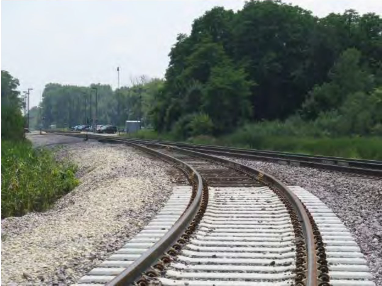
Figure 2-145. Junction of Zion On-site Rail Spur with Union Pacific Railroad Showing Concrete Rail Ties (2013)
