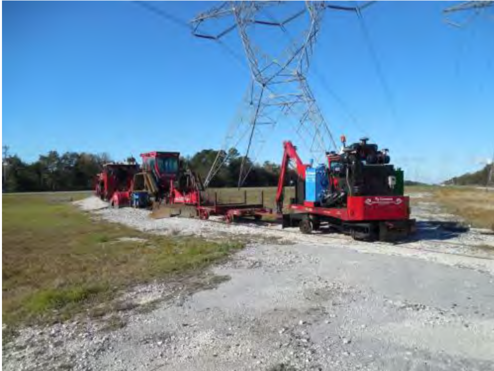
Figure 2-173. Track Maintenance Equipment Staged at the Mine Spur (2015)
