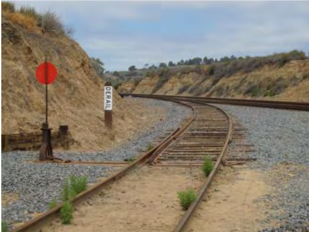
Figure B-57. North County Transit District Split Rail Derailer (2015)
