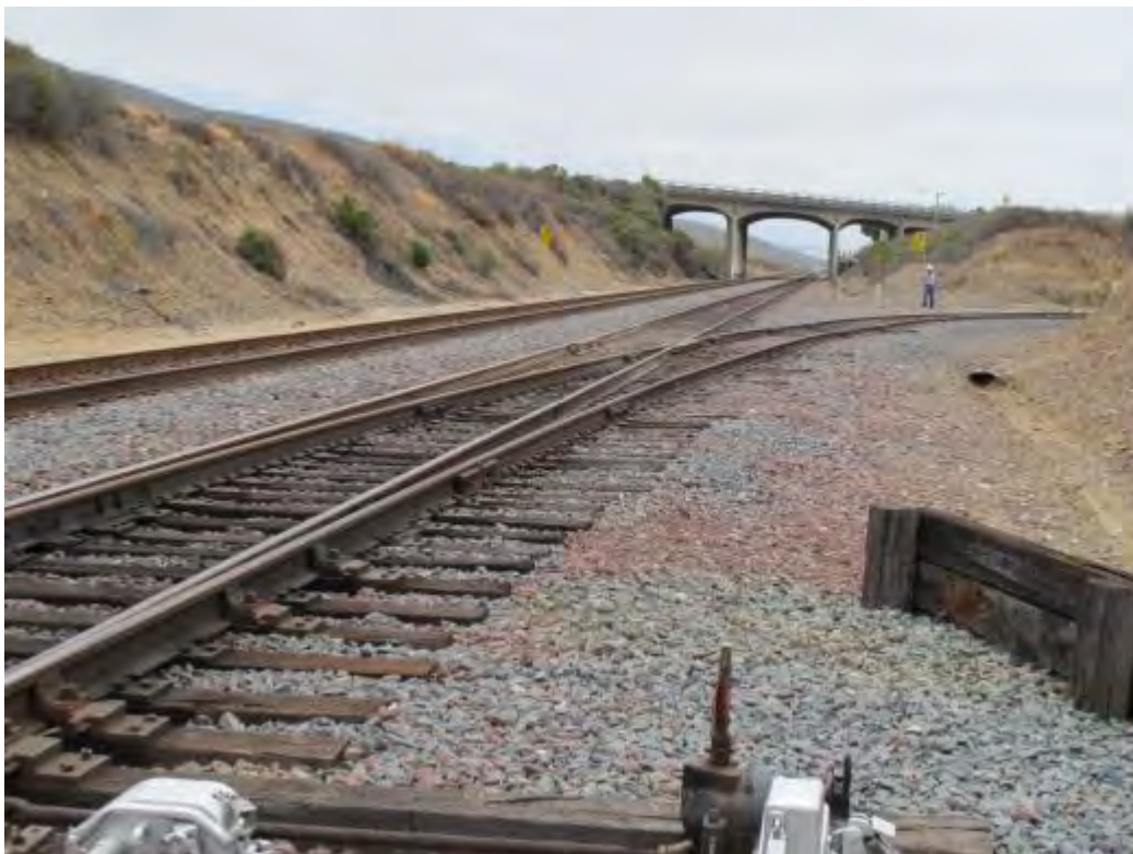
Figure 2-285. Mainline at San Onofre Site (Looking South) (2015)
