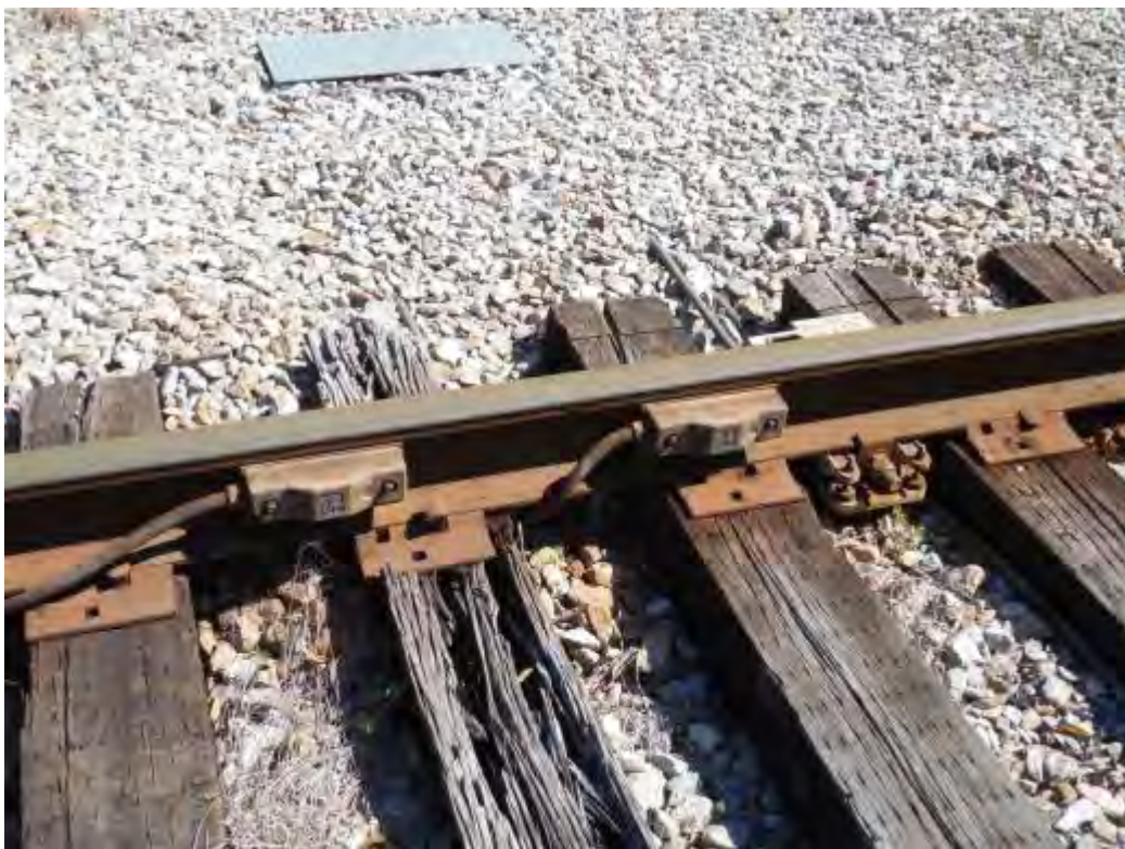
Figure 2-170. Wheel Detectors on Florida Northern Railroad (2015)
