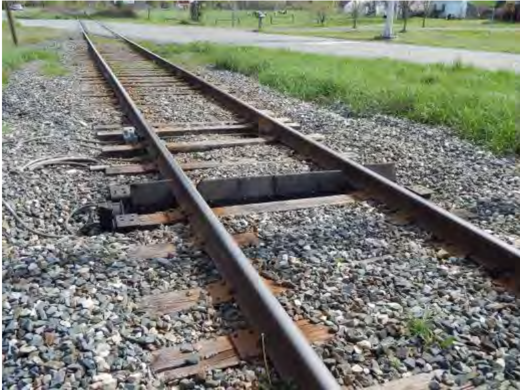
Figure 2-317. Dragging Equipment Detector and Hot Bearing Detector on New England Central Railroad Mainline (2016)
