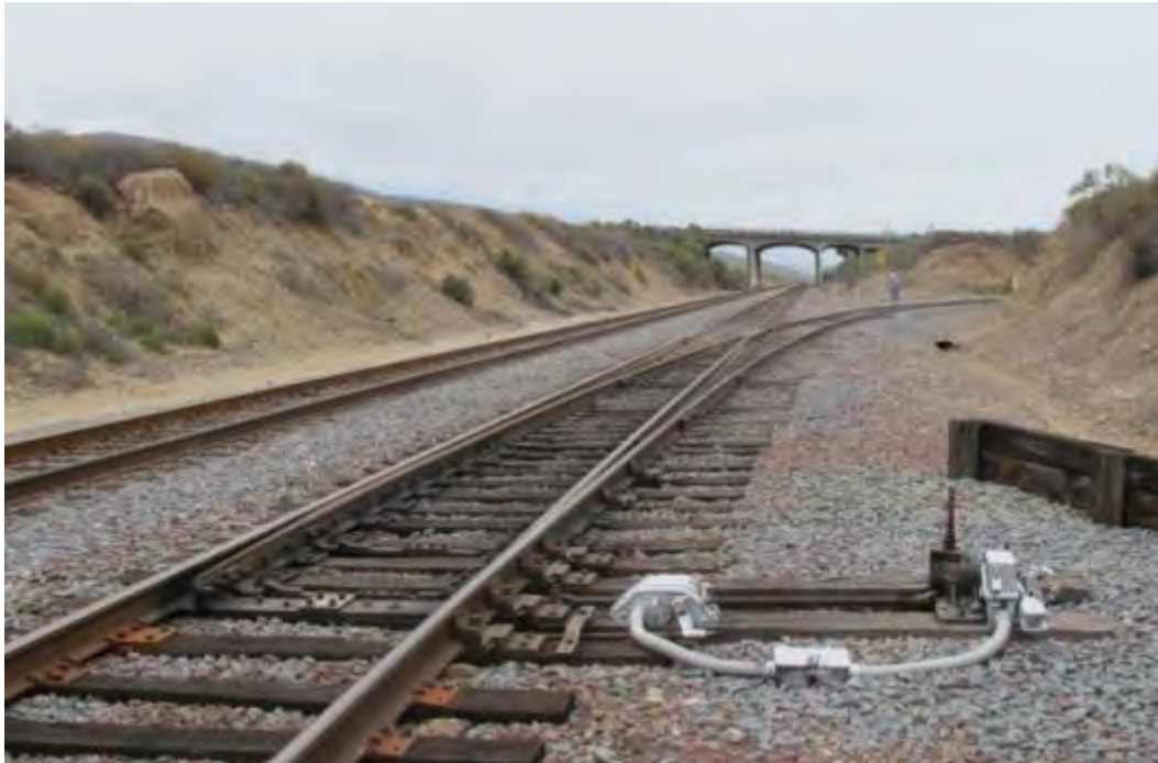
Figure B-56. Manually Operated, Timed Switch (2015)
