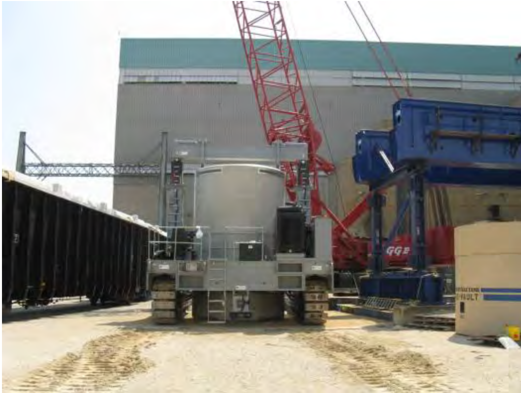
Figure 2-139. Transporter Used to Move Vertical Concrete Storage Casks (2013)
