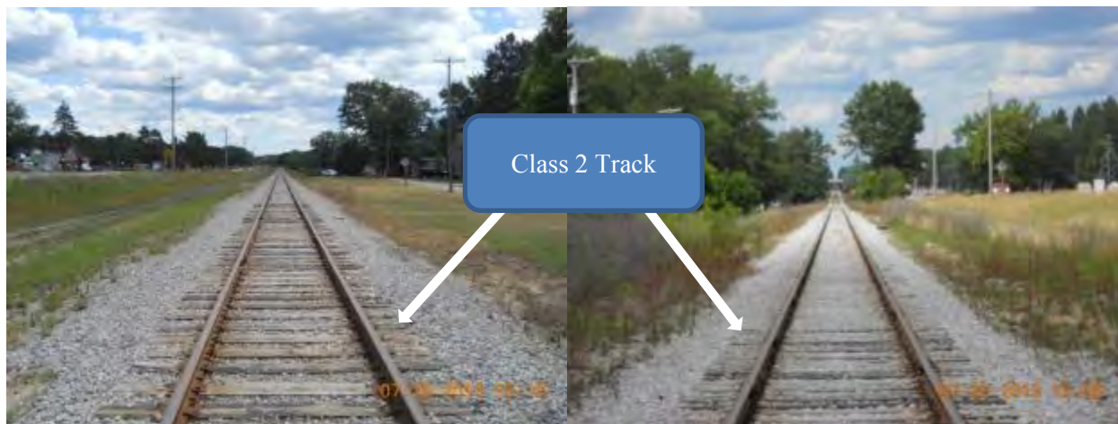
Figure B-9. Track Condition in the Vicinity of Gaylord Transload Location (Looking South) (2013)
