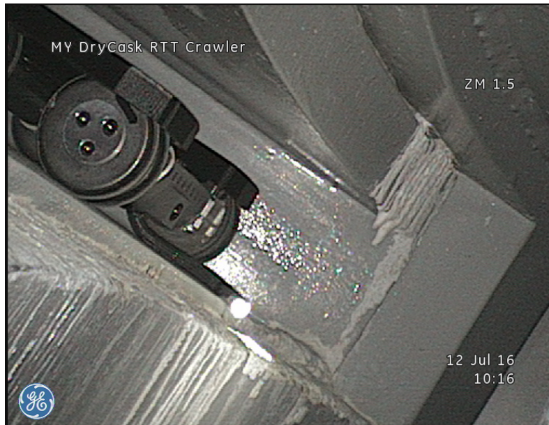
Figure 12. Video image of white crusts of cementitious material on the inner surface of the overpack, located near an outlet vent.
