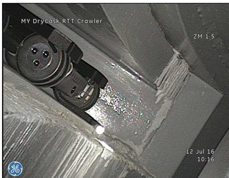
Figure 29. Video image of white crusts of cementitious material on the inner surface of the overpack, located near an outlet vent.
