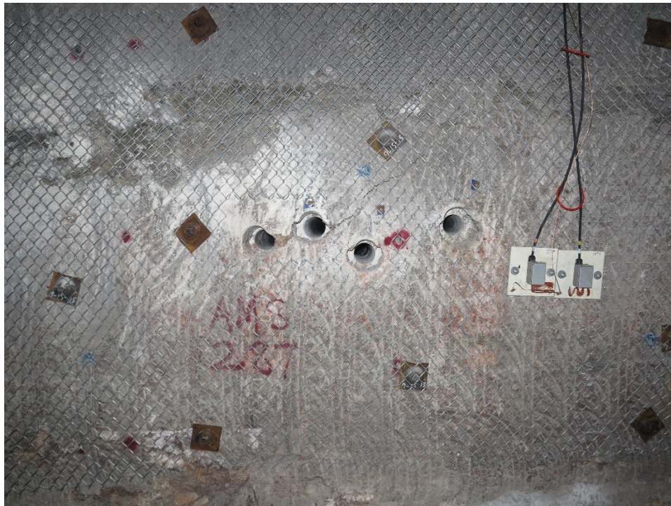
Figure 2. Configuration of existing boreholes used in Phase 1 testing. SNLCH111 is the right most 12 cm boreholes and numbering increases to the left.
