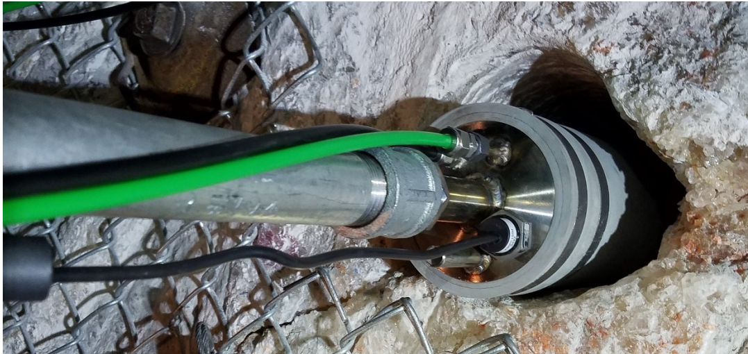
Figure 7. Pre-assembly test of Phase 1 packer system used to isolate the heated borehole from the access drift.
