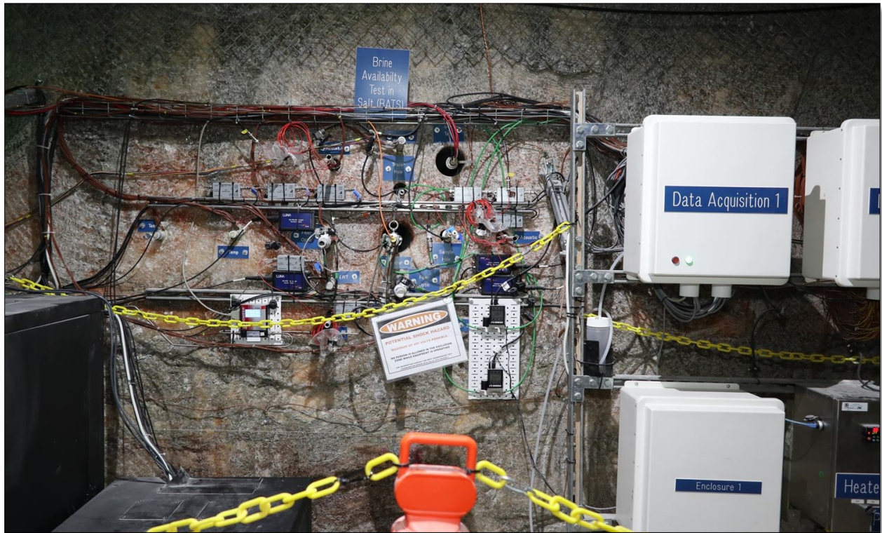
Figure 4. BATS test (heated array) in December 2019
