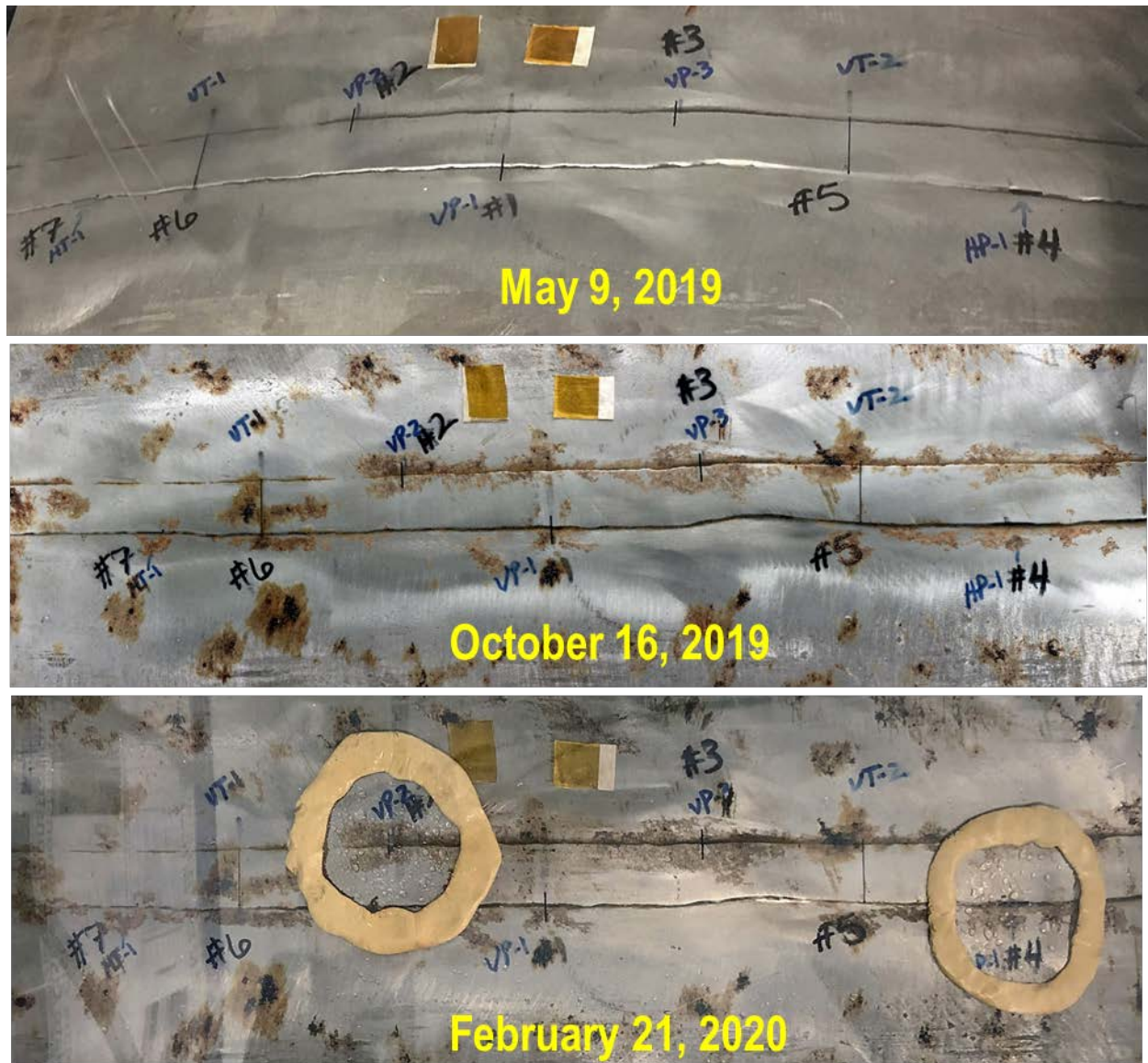
Figure 14. Evolution of general corrosion on the large plate in weld region
