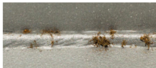
Example of pitting corrosion at a weld
