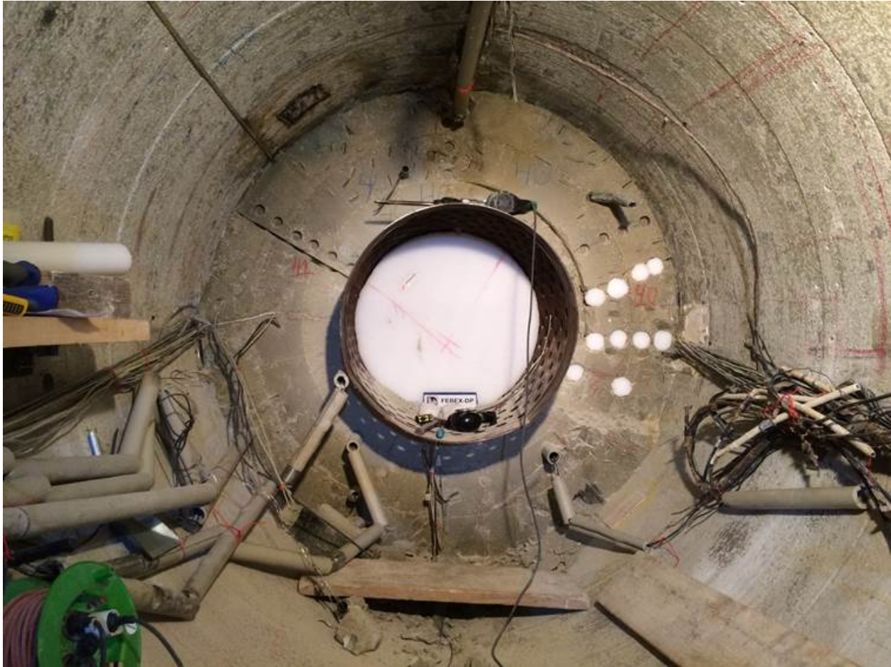
Figure 1. Exposure face of FEBEX experiment during dismantling of experiment. Note steel liner near center and Grimsel granodiorite at outer edge of drift.
