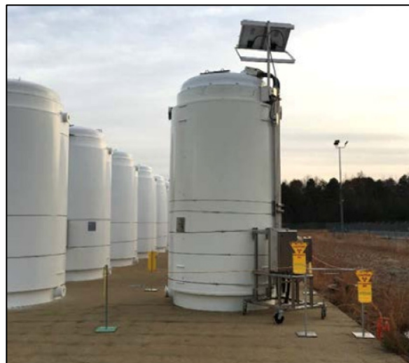
Figure 2. TN-32B HBU demonstration cask on North Anna ISFSI and temperature data equipment (Photo courtesy of Dominion Energy).
