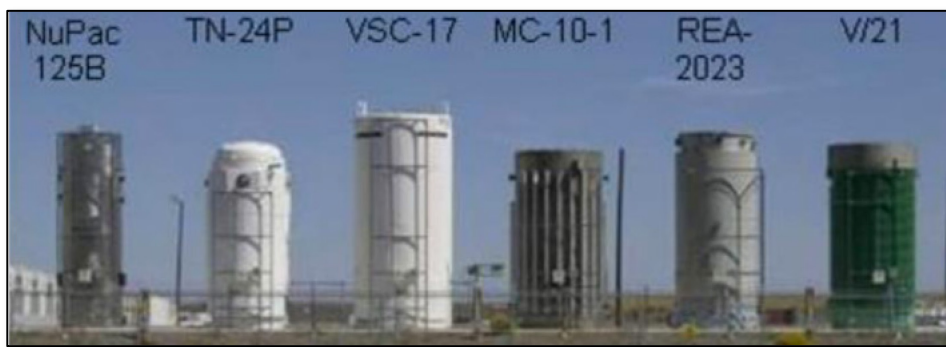
Figure 14. Six of eight casks on CPP-2707 cask pad.
