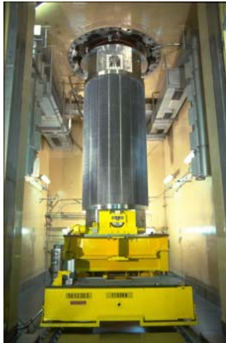
Figure 8-16. Dry Transport Canister Attached to Dry Unloading Cell
