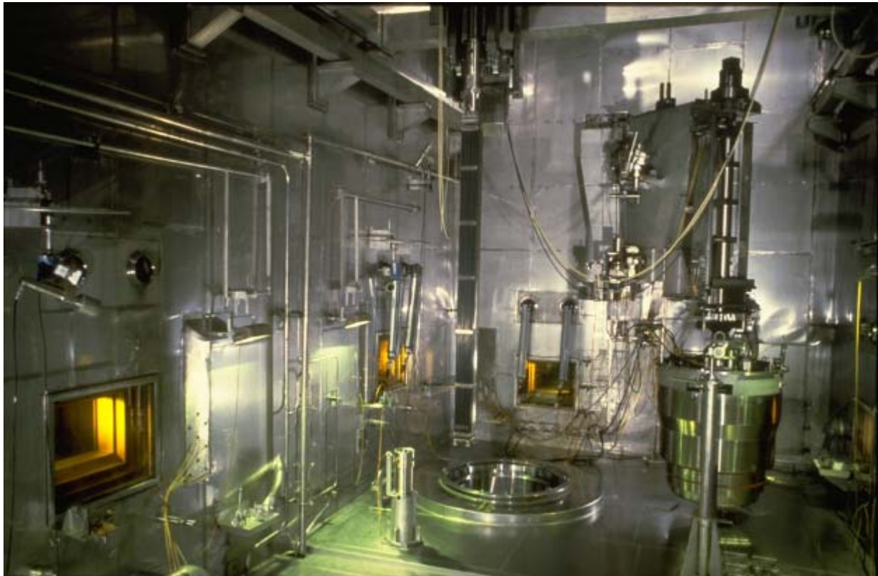
Figure 8-17. View Inside T(0) Dry Unloading Cell with Final Canister Plug Removed
