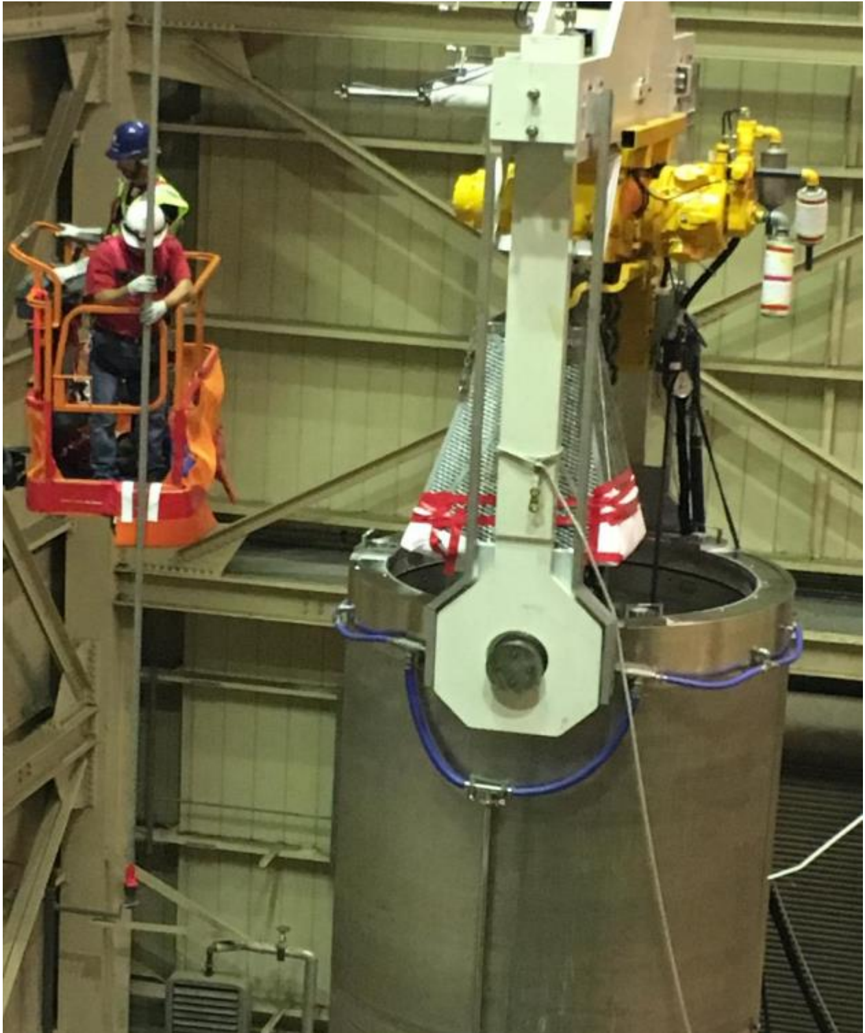
FIGURE 2-31: MAGNASTOR TRANSFER CASK [41] ENGAGED TO SECURE-LIFT YOKE
