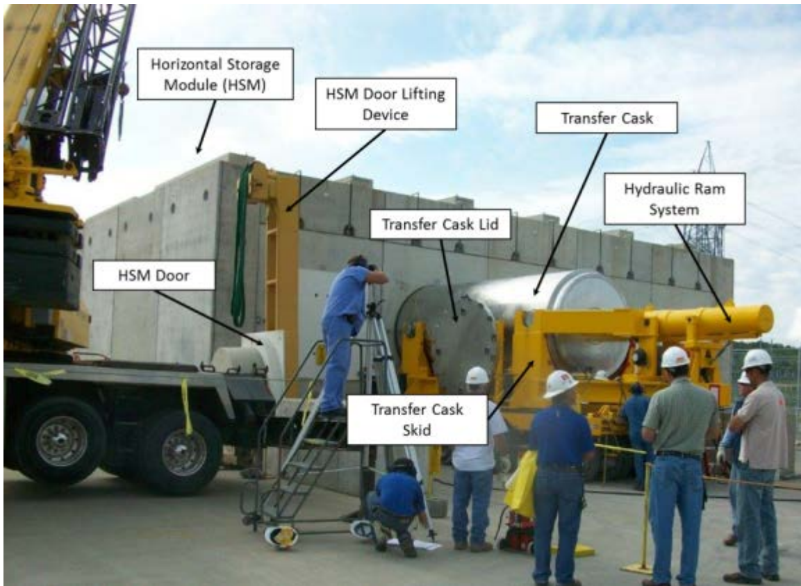
FIGURE 2-13: DOCKED NUHOMS TRANSFER EQUIPMENT
