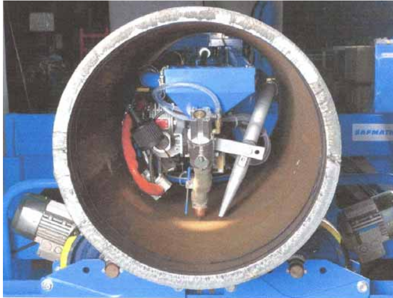
Figure 5.2.21 Welding robot used for welding inside the sleeve (photograph courtesy of Air Liquide)
