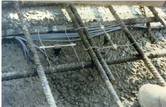
Figure 10.3.1 Illustration of a vibrating wire extensometer, attached to a reinforcement and integrated in the concrete structure
