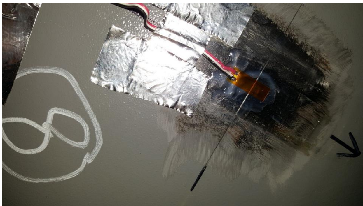
Figure D12. SGBF8 LH side of Bottom Flange of Center Sill, aft of Front Body Bolster, aligns with Center Sill Web and End Stop Mount Block Pin Hole
