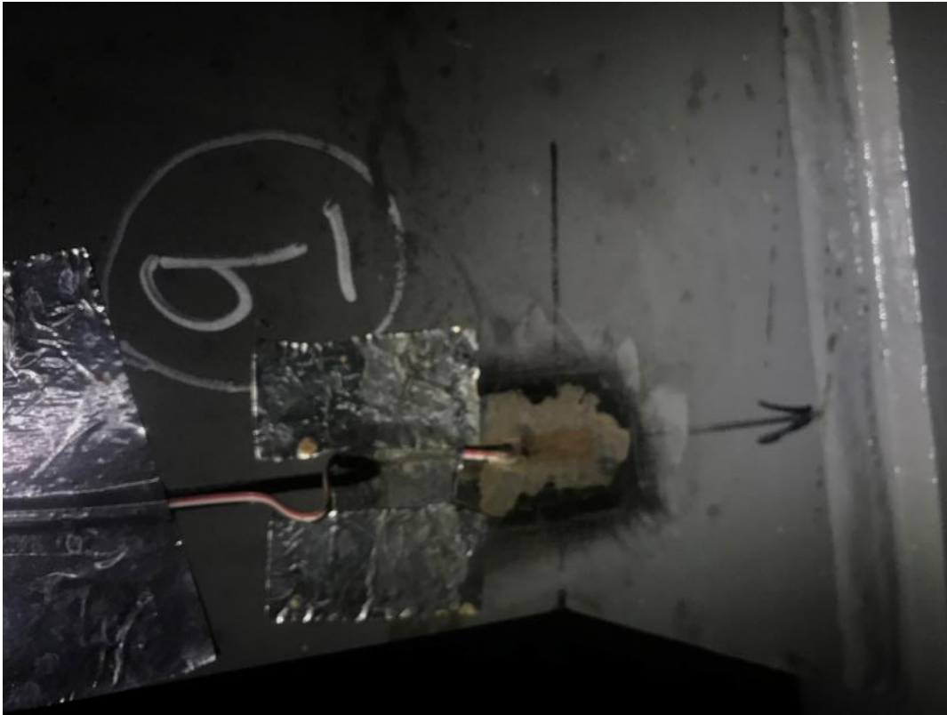
Figure D13. SGBF9 Front of Bottom Flange of #4 Cross Bearer, LH Side between Center Sill and Side Sill, near Center Sill
