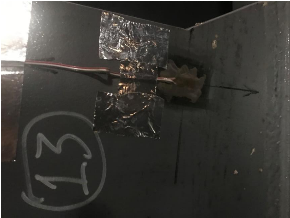
Figure D17. SGBF13 Rear of Bottom Flange of #4 Cross Bearer, LH side between Center Sill and Side Sill, near Center Sill
