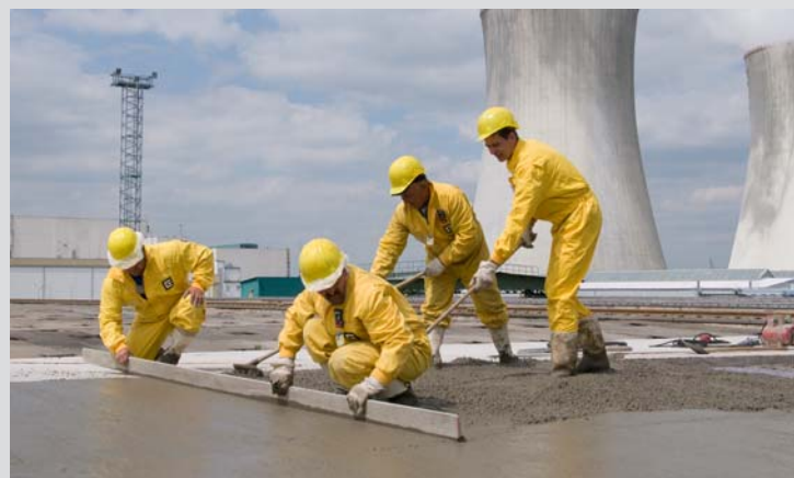
Finalising the closure of the vault by the laying of concrete over the surface of the panels.
