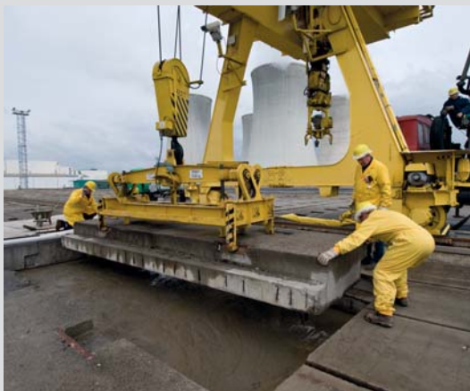
Sealing of a filled vault; the space between individual drums has been filled with concrete.
