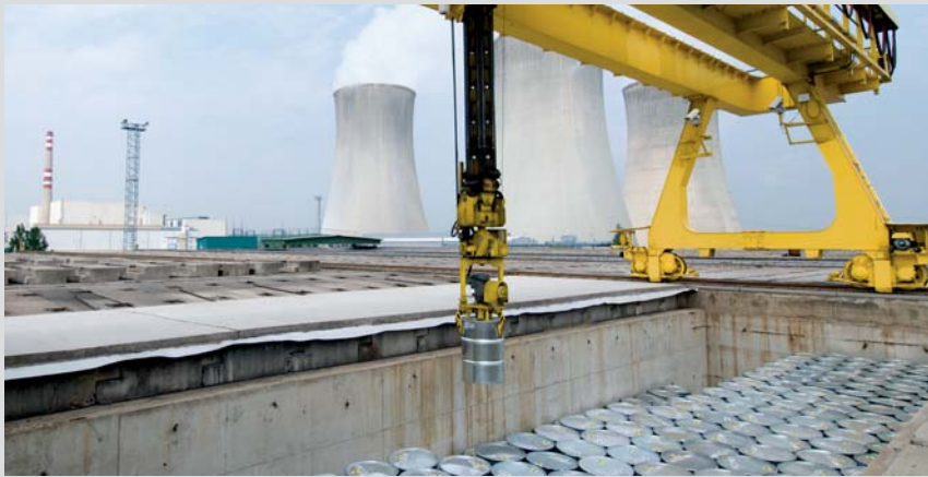
Placement of radioactive waste in an emplacement vault at the Dukovany repository.
