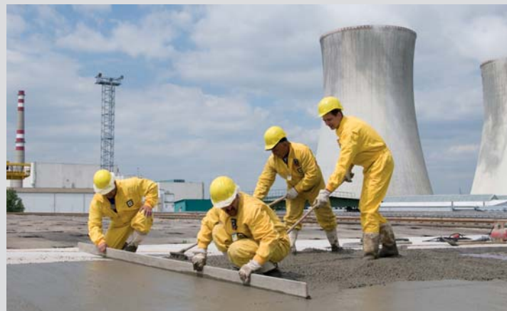
Completion of the temporary insulation of a filled vault (a final overlay will be added before repository closure).
