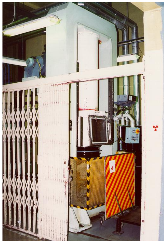
Waste compressor machine
