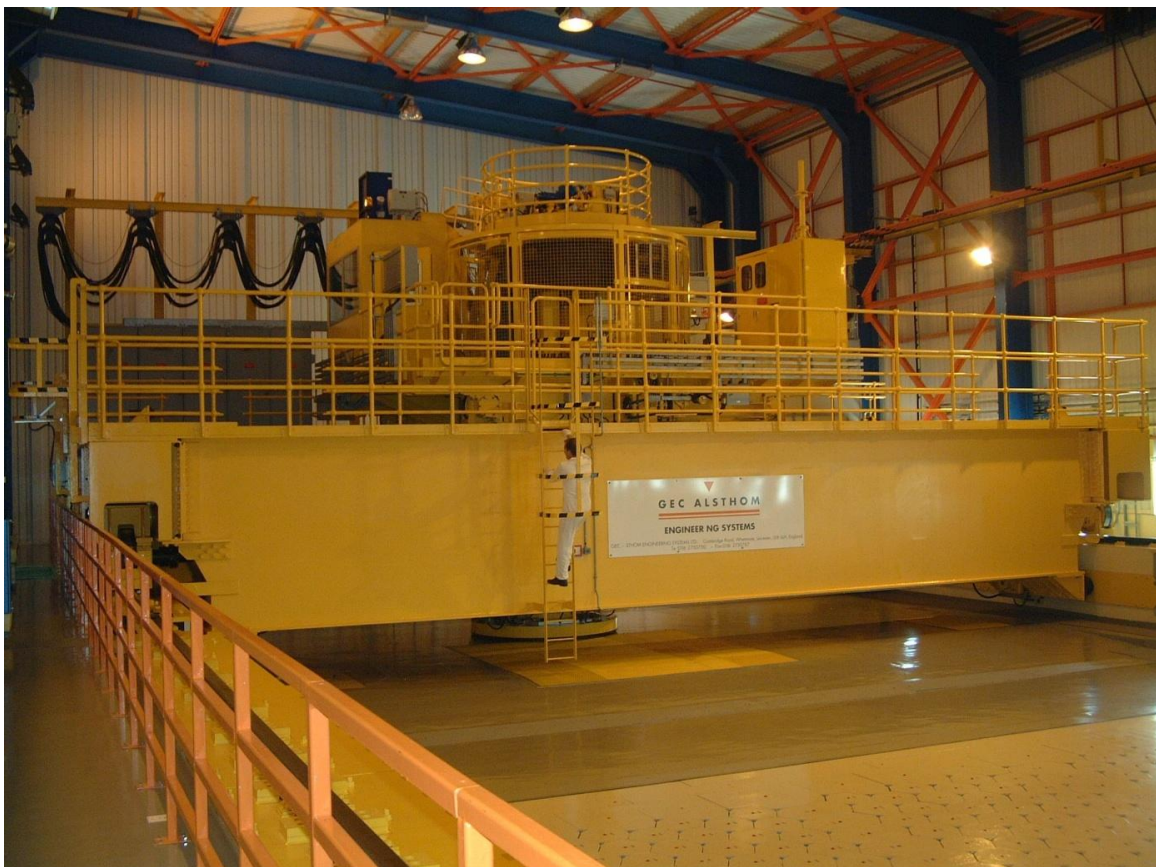
Re-fuelling machine in the Interim Spent Fuel Storage Facility
