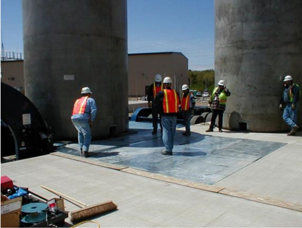
Figure 2-30: NAC VCC Movement to/from ISFSI Pad on Air Pads
