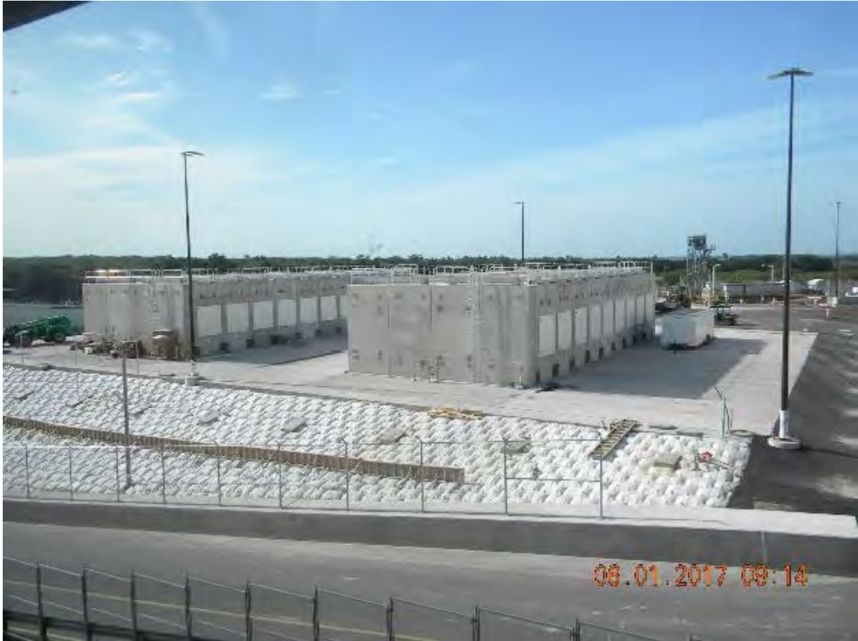
Figure 2-6: Crystal River Independent Spent Fuel Storage Installation with Horizontal Storage Modules Installed 121
