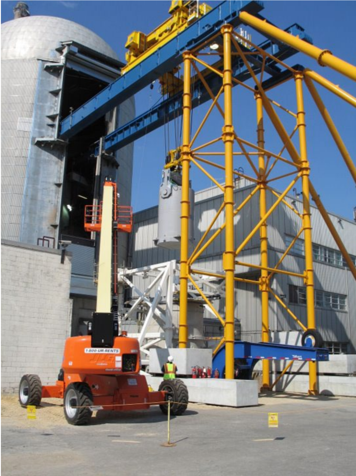
Figure 2-30: MPC-LACBWR TFR Moving to Transfer Position on VCC and TFR Restraint System
