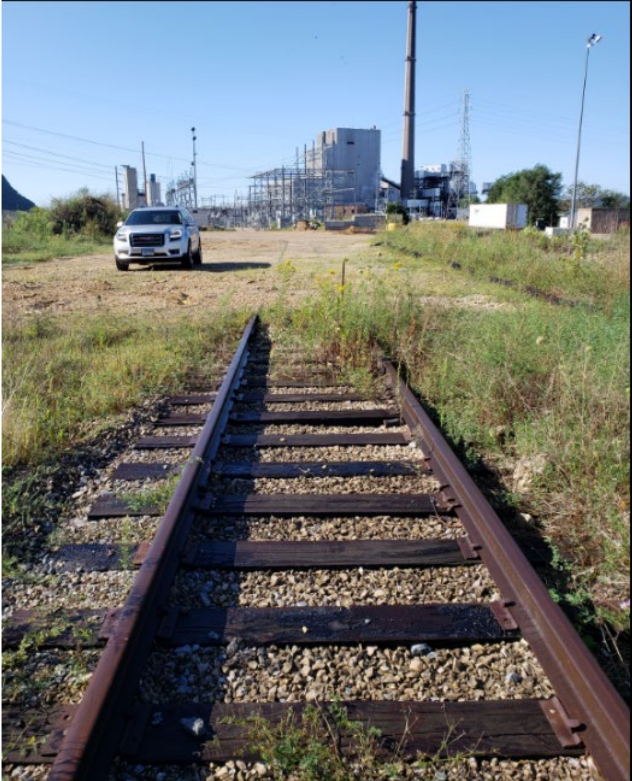
Figure 2-13: On-Site Rail Spur South View
