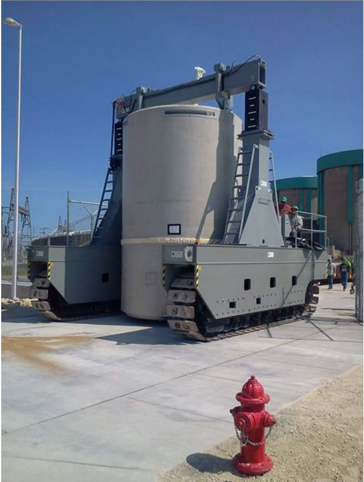
Figure 2-18: MAGNASTOR Loaded Zion VCC Transferred to the ISFSI by VCT [20]
