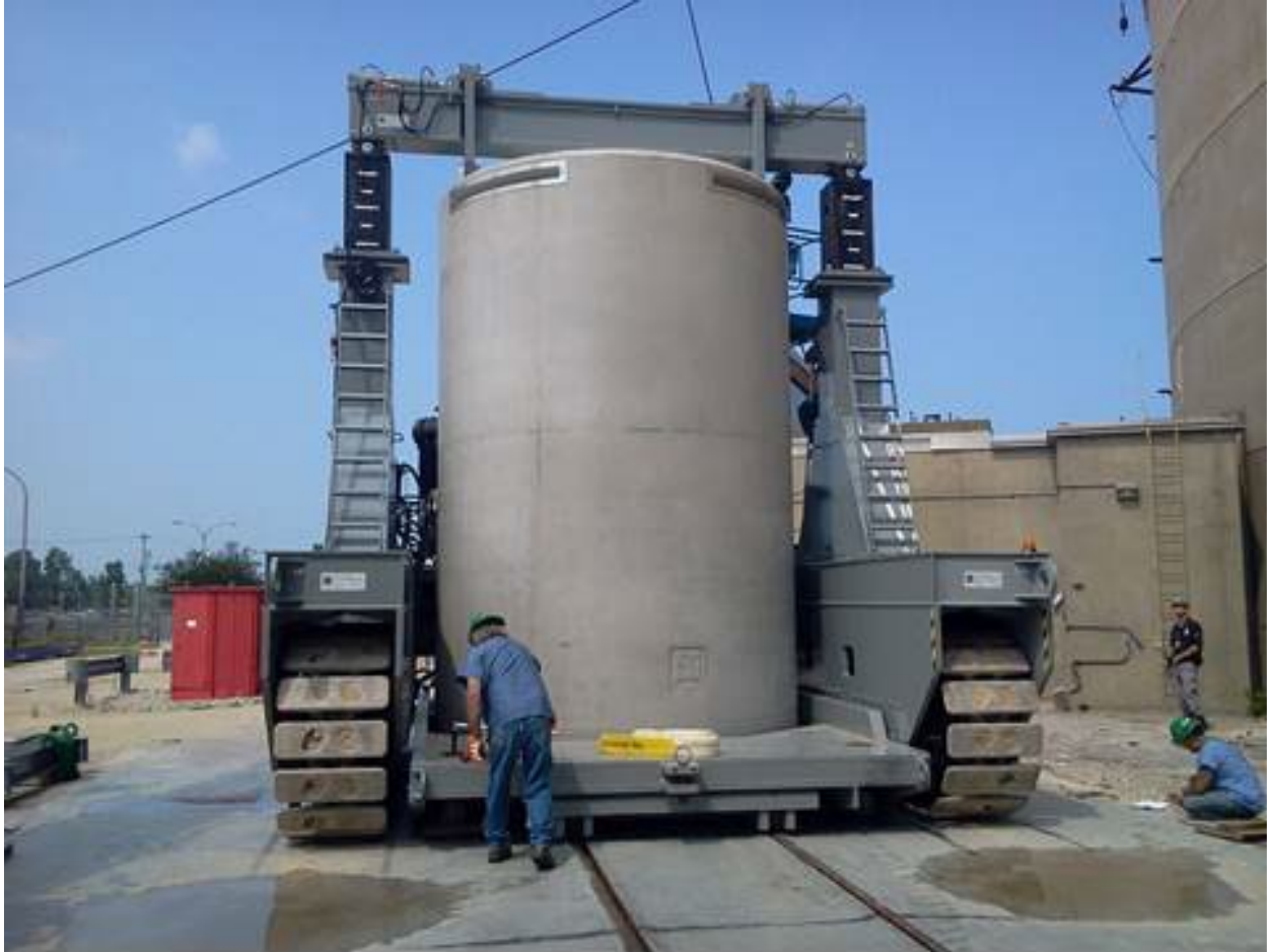
Figure 2-17: MAGNASTOR Vertical Zion VCC Engaged to VCT and Being Removed from LPRC
