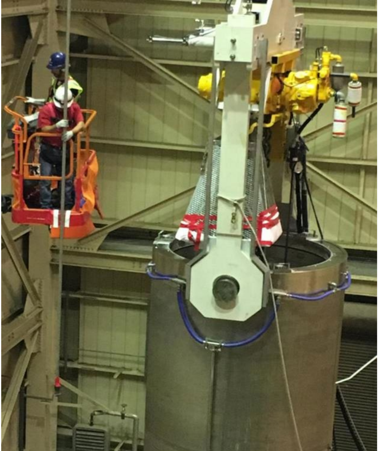
Figure 2-33: MAGNASTOR Transfer Cask [19] Engaged to Secure-Lift Yoke
