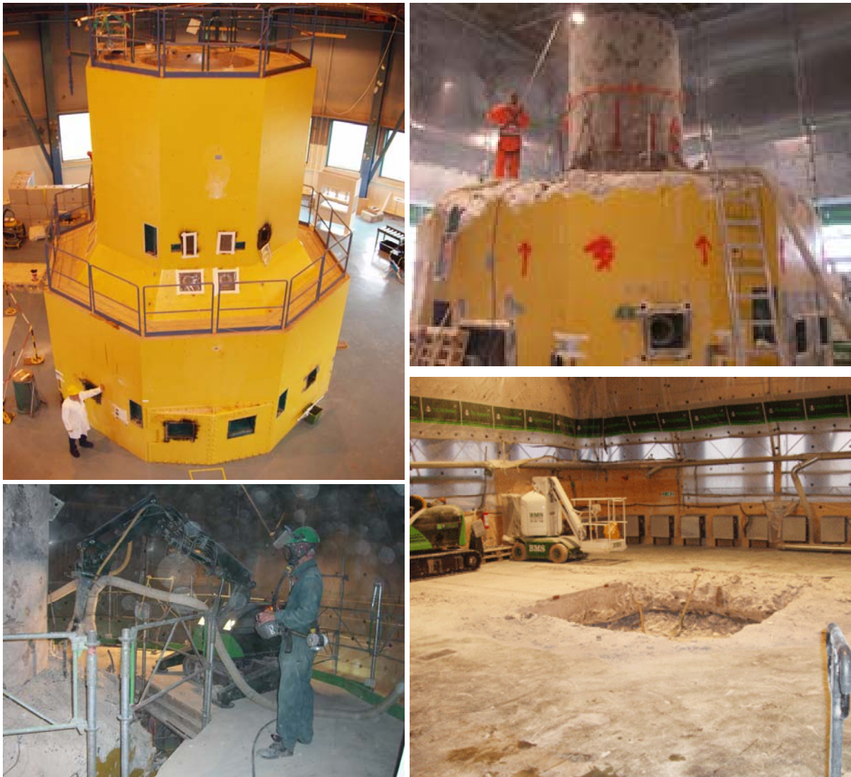
Figure 3, (Upper left) DR 2 from above, (upper right) Destruction of concrete shield, to avoid spreading of dust a tent, with low pressure inside, was raised around the reactor, (lower left) Destruction of DR 2 reactor block, (lower right) After the reactor block is removed only a 16 m 2 hole remains.
