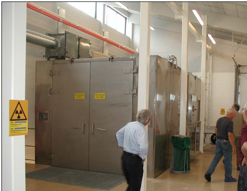
Figure 2. Decontamination cabinet for high pressure water or glass blasting.
