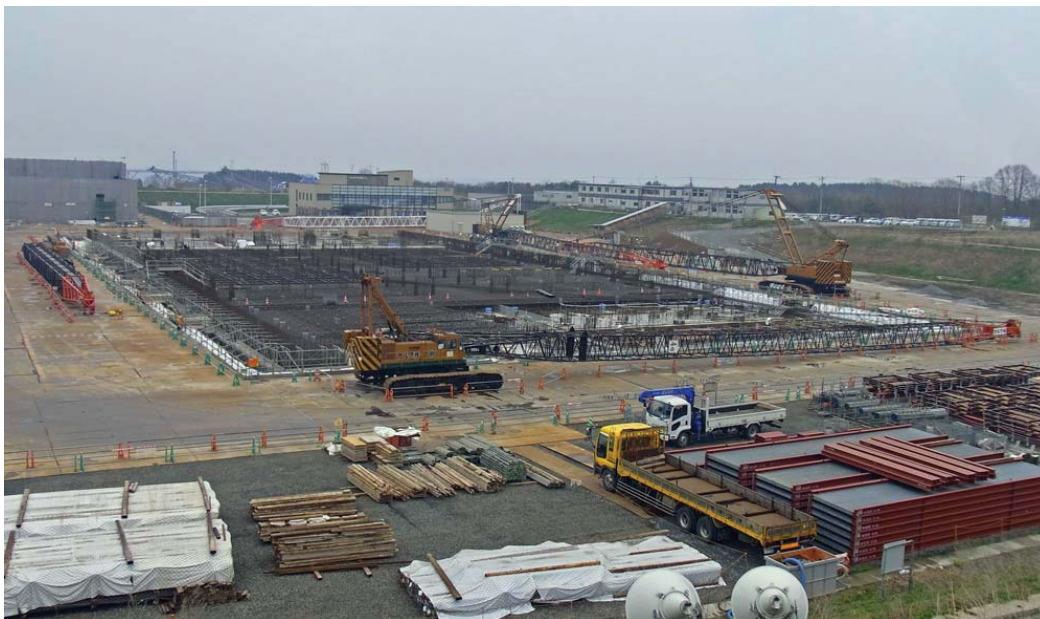
Fig. L5-2 Construction site view of Recyclable-Fuel Storage Center (Source: Home page of Recyclable-Fuel Storage Company)
