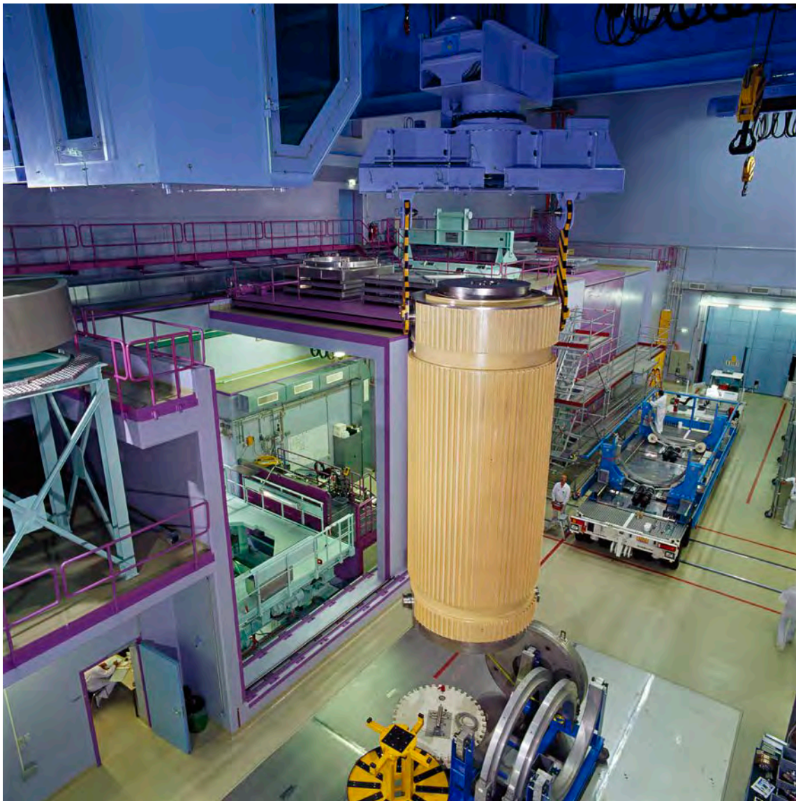
Figure 14: Reception of a transport cask with radioactive waste from reprocessing in ZZL (Photo: Zwiilag)
