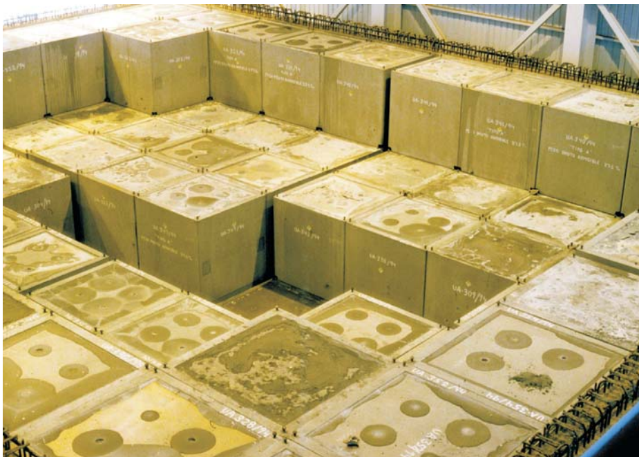
Radioactive waste management facilities: disposal of containers in cells (El Cabil).
