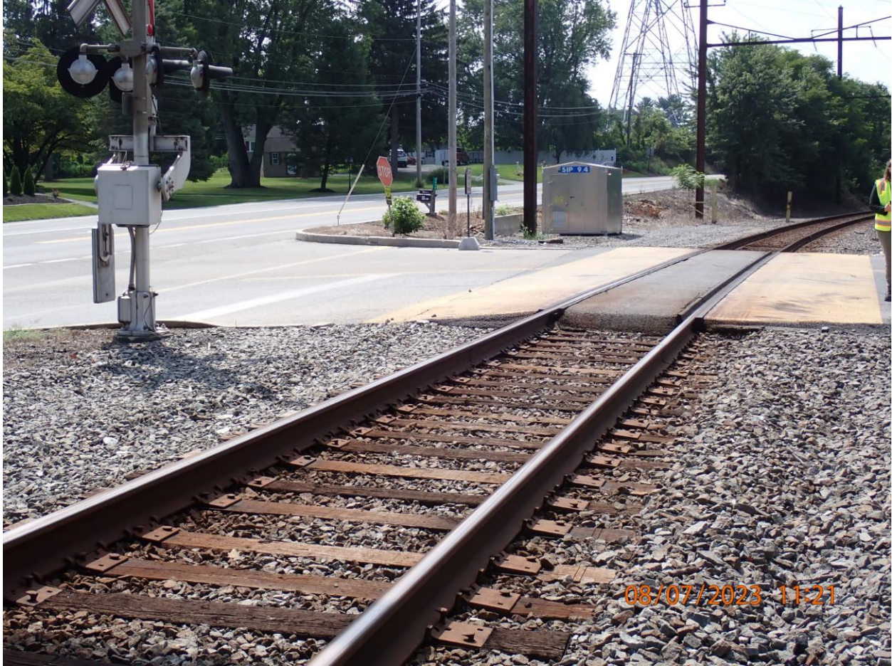
Figure 15. Norfolk Southern Rail Line at Entrance to the Three Mile Island Site
