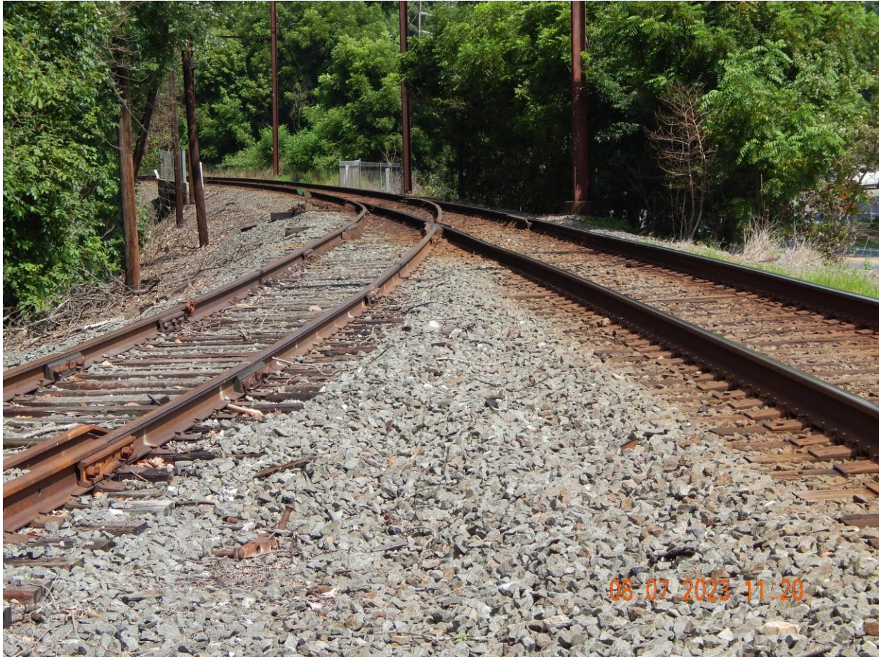
Figure 14. Three Mile Island Onsite Rail Spur Approaching Norfolk Southern Rail Line
