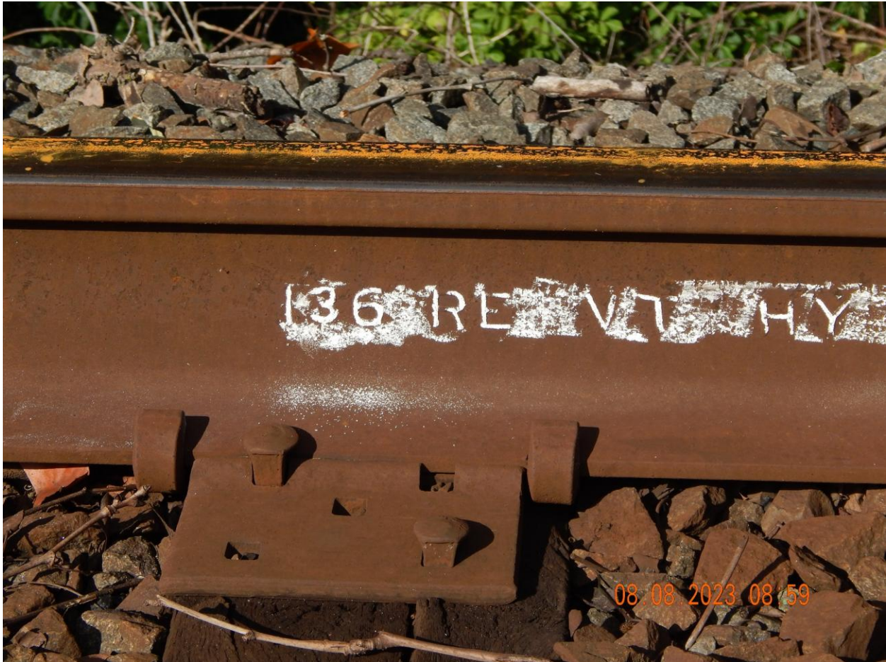
Figure 17. Norfolk Southern 136-lb Rail at Entrance to the Three Mile Island Site
