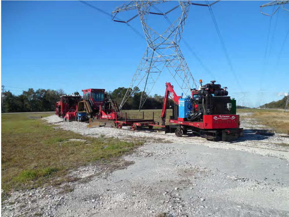
Figure 2-177. Track Maintenance Equipment Staged at the Mine Spur (2015)
