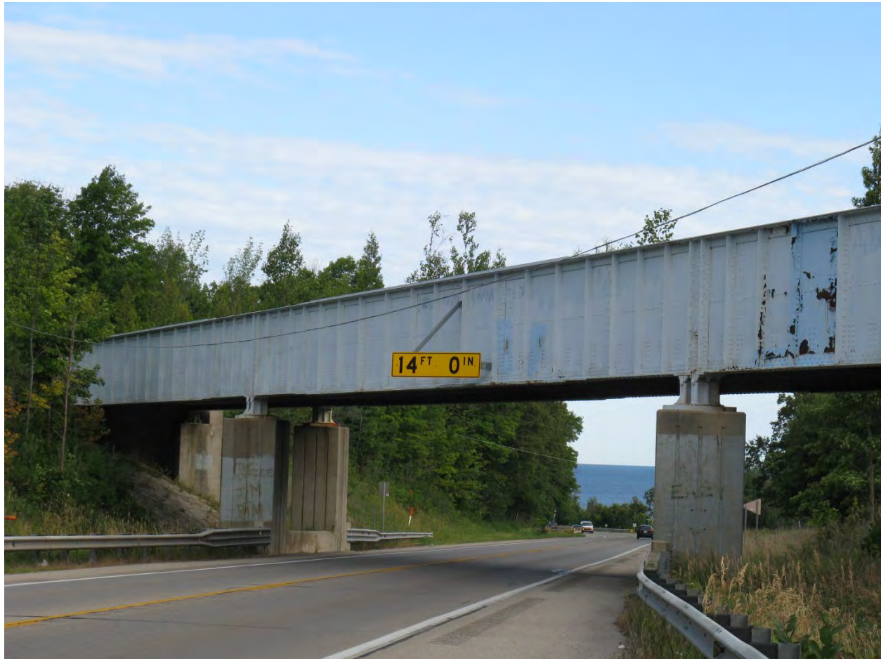
Figure 2-75. Low Overhead Clearance Abandoned Railroad Bridge on U.S. 31 (2013)
