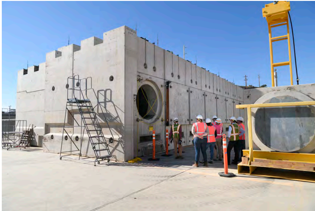
Figure 2-279. Open Reinforced Concrete Horizontal Storage Module and Shielded Access Door (2022)
