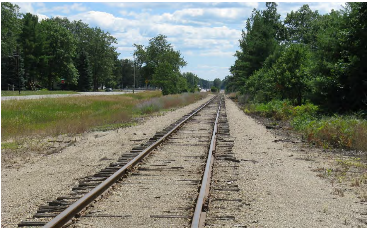
Figure 2-78. Condition of Rail Crossing Used for Big Rock Point Reactor Pressure Vessel Transload (Looking South) (2013)
