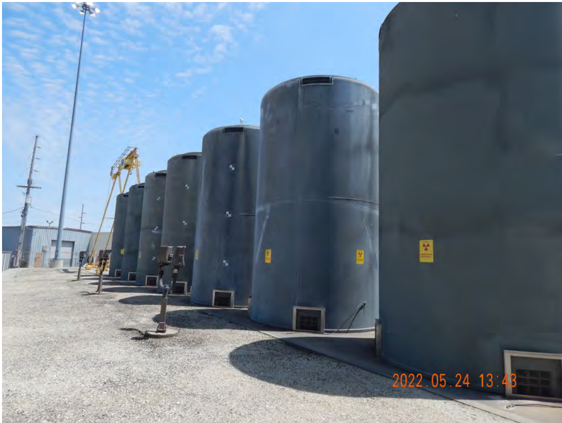
Figure 2-445. HI-STORM Dry Storage Systems at East ISFSI
