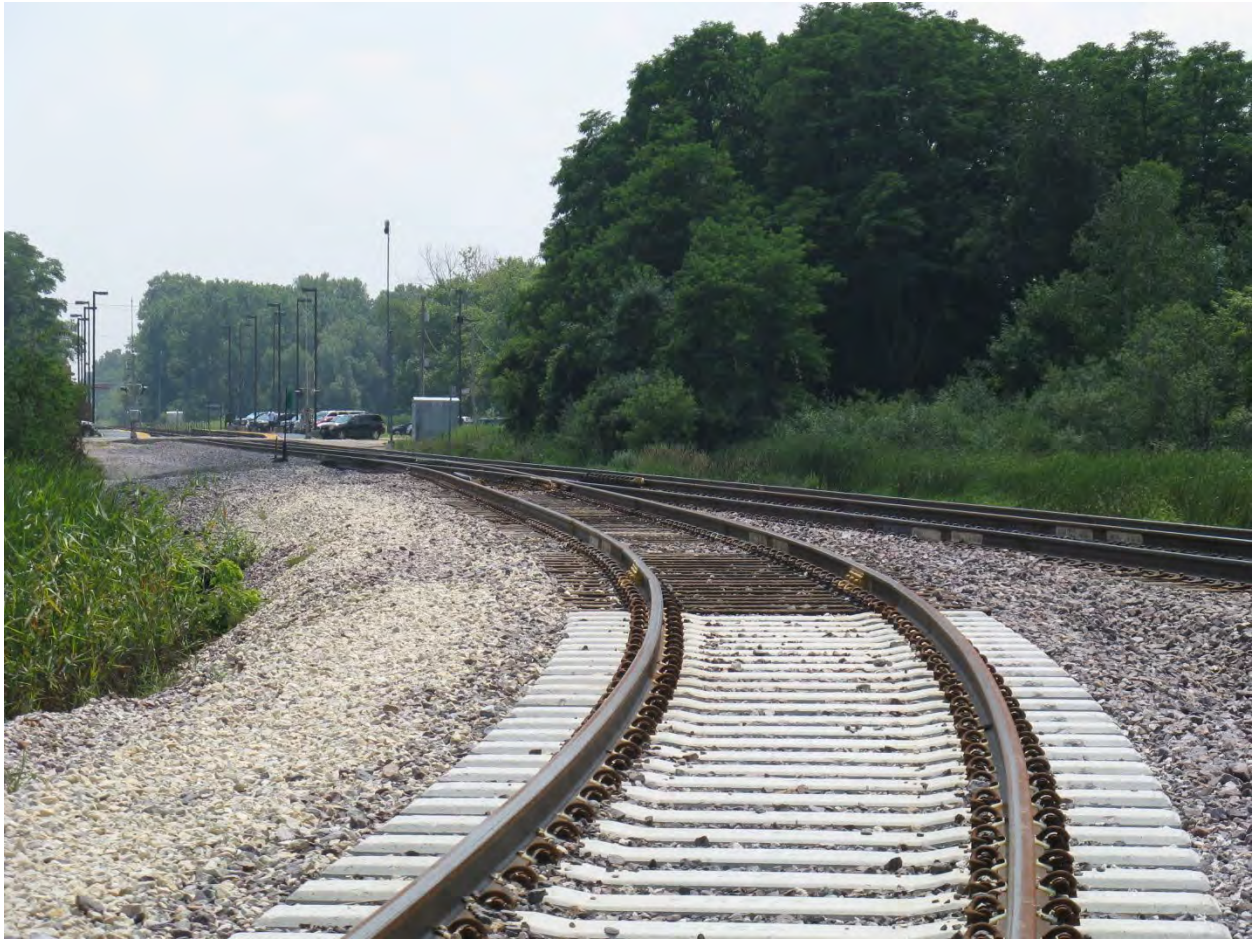
Figure 2-147. Junction of Zion On-site Rail Spur with Union Pacific Railroad Showing Concrete Rail Ties (2013)
