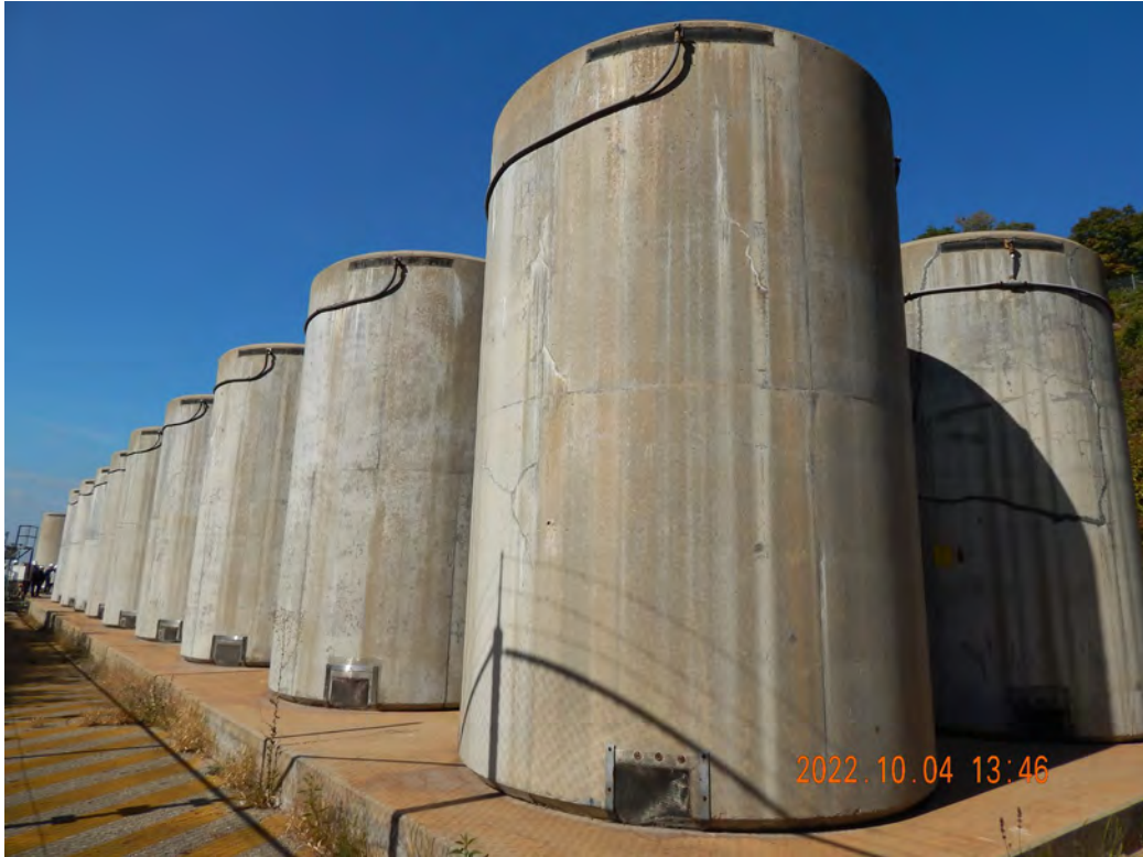
Figure 2-573. VSC-24 Dry Storage Systems at the Original ISFSI Looking West
