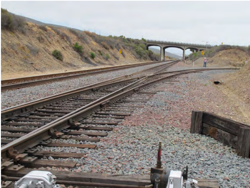
Figure 2-302. Mainline at San Onofre Site (Looking South) (2015)
