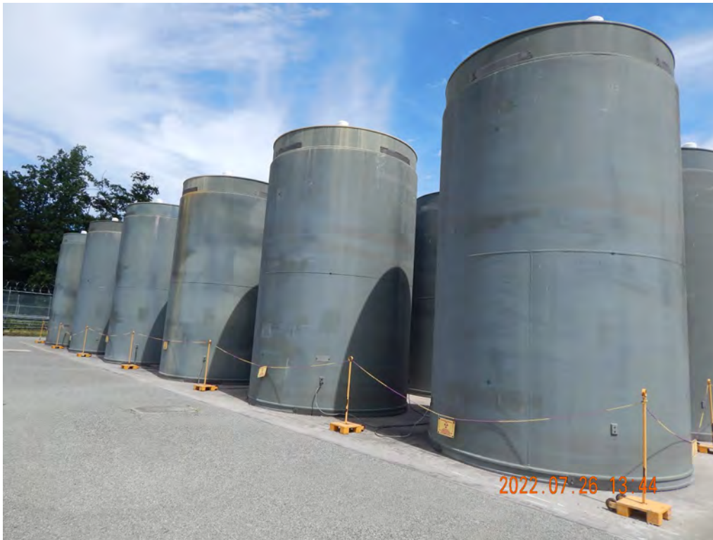
Figure 2-512. HI-STORM FW Dry Storage Systems at the Indian Point ISFSI (Looking North)
