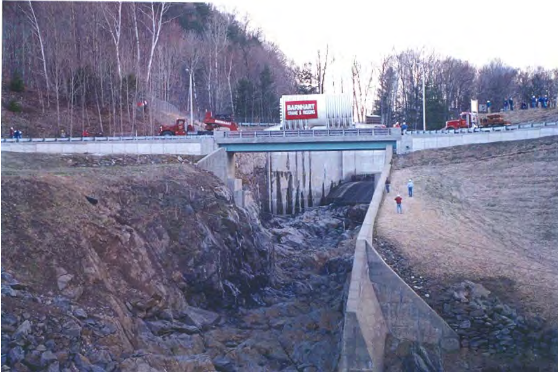
Photo courtesy of AREVA
