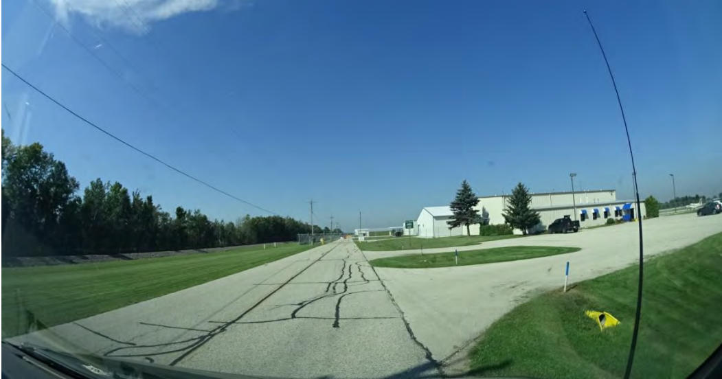
Figure 2-240. Access Road at Potential Rockwood Spur at the Manitowoc Airport Transload Location (Looking North) (2014)
