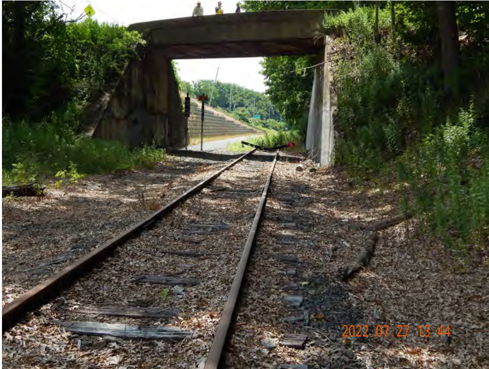
Figure 2-551. State Line Potential Transload Location Looking Southwest at Cut Rail at CT-NY Border
