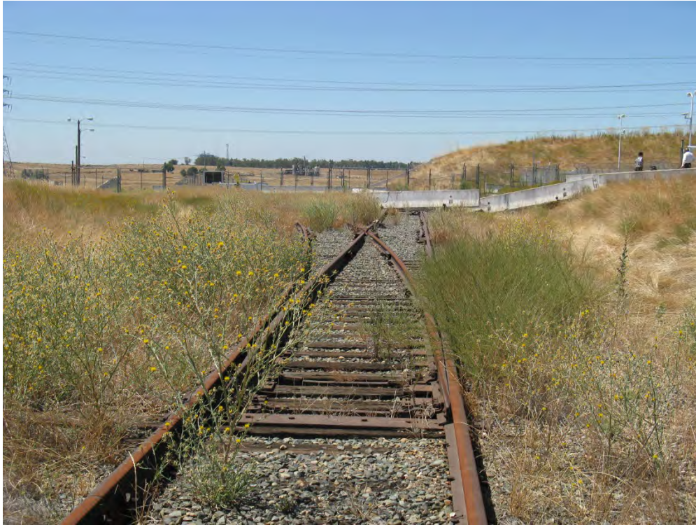
Figure 2-91. Junction of the On-site Track Spur Running Adjacent to the Independent Spent Fuel Storage Installation (Right) and the Longer Track Running into the Rancho Seco Site (Left) (2013)
