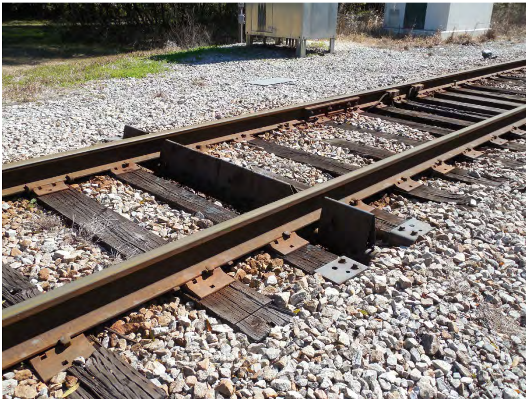
Figure 2-176. Dragging Equipment Detector on Florida Northern Railroad (2015)
