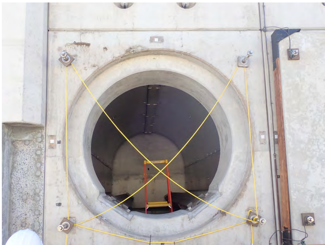
Figure 2-280. Interior of Open Reinforced Concrete Horizontal Storage Module (2022)
