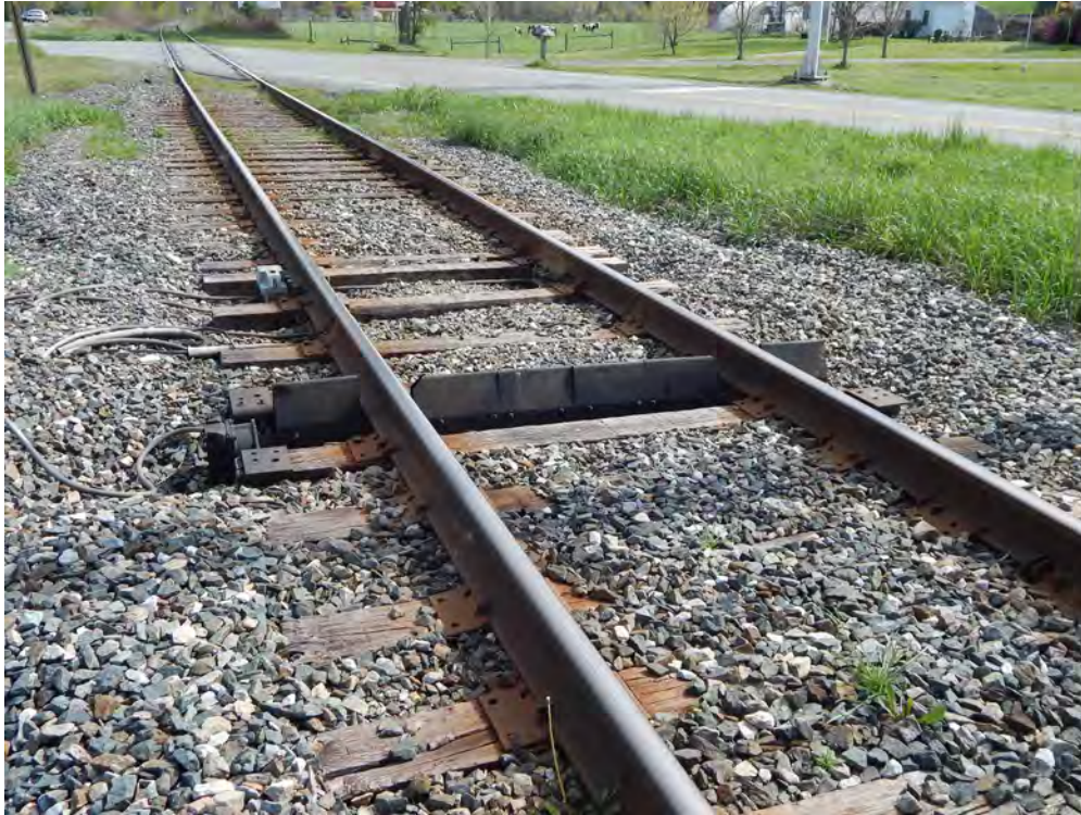
Figure 2-331. Dragging Equipment Detector and Hot Bearing Detector on New England Central Railroad Mainline (2016)
