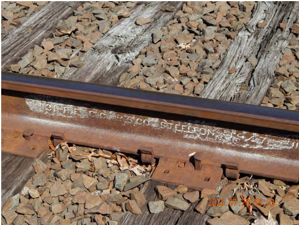
Figure 2-534. 131-lb. Rail Hawleyville Road Potential Transload Location
