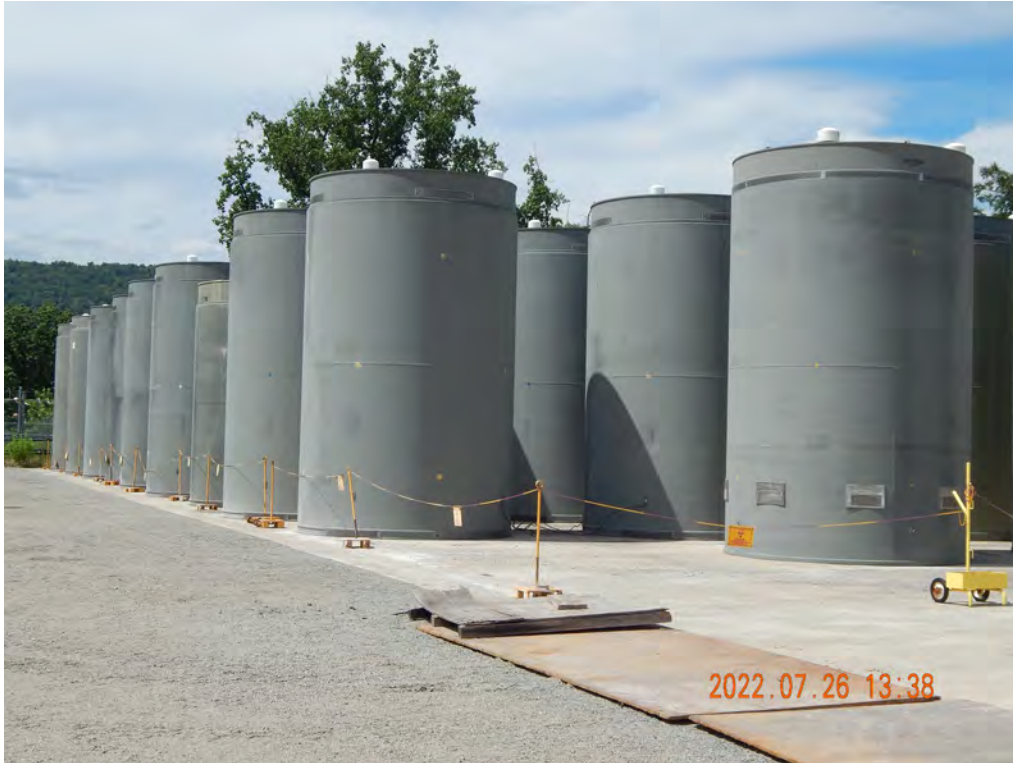
Figure 2-511. HI-STORM FW Dry Storage Systems at the Indian Point ISFSI (Looking West Towards Hudson River)
