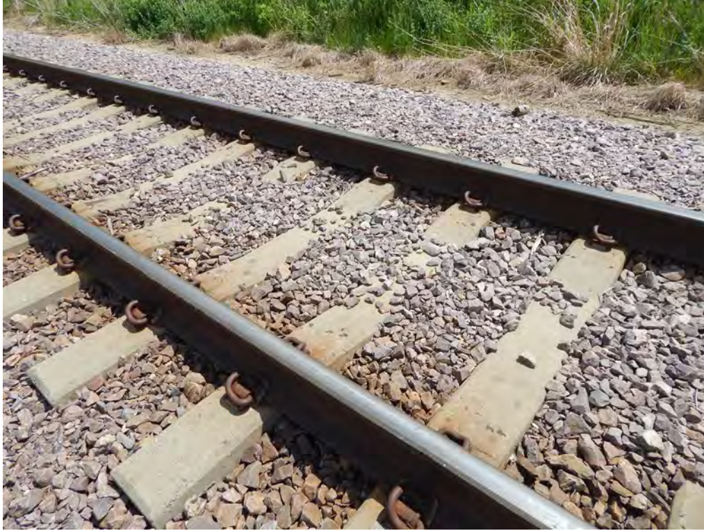
Figure 2-350. Rail, Concrete Ties, and Pandrol Clips on Cargill Industrial Spur (2017)
