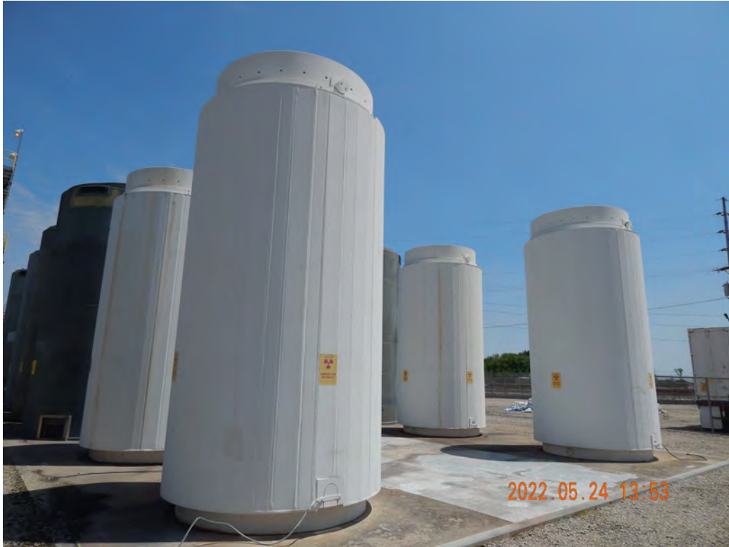
Figure 2-446. HI-STAR 100 Dry Storage Systems at East ISFSI
