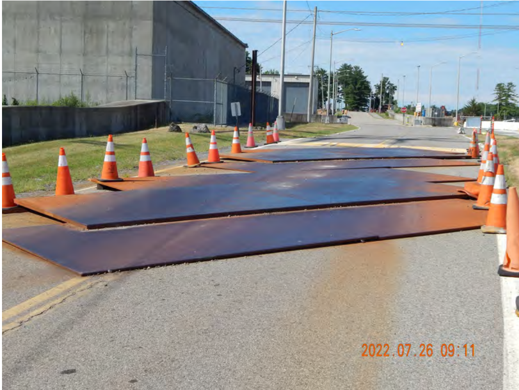
Figure 2-525. Air Bridge Over 26-inch and 30-inch Gas Lines Looking South
