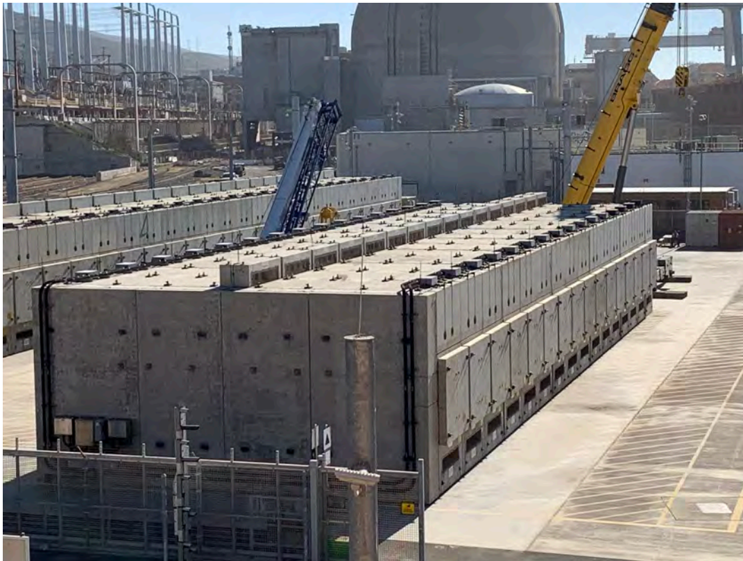
Figure 2-276. Original San Onofre Independent Spent Fuel Storage Installation (2022)
