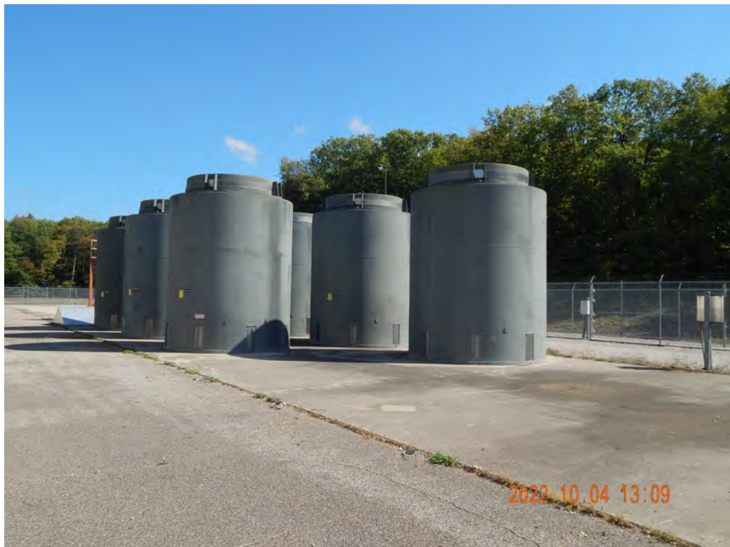
Figure 2-576. HI-STORM FW Dry Storage Systems at the East ISFSI at the Palisades Site
