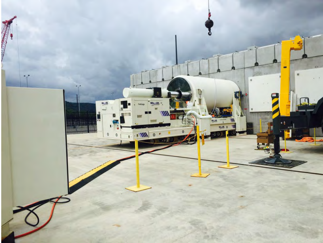
Photo courtesy of AREVA TN
