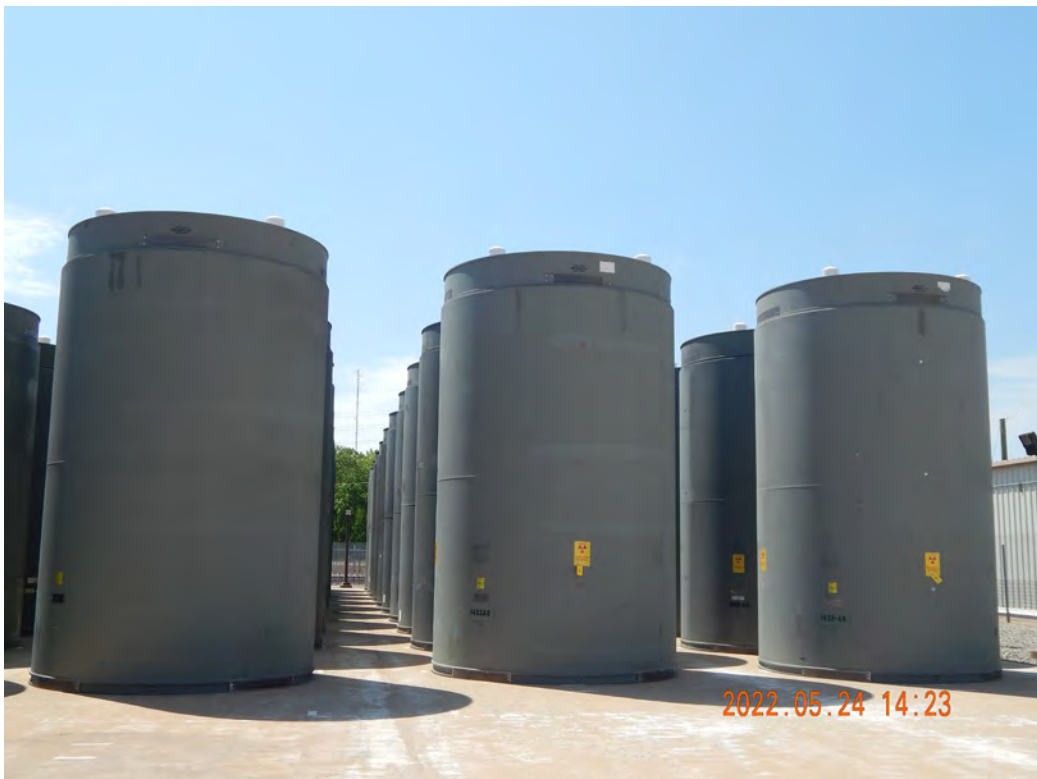
Figure 2-447. HI-STORM Dry Storage Systems at West ISFSI
