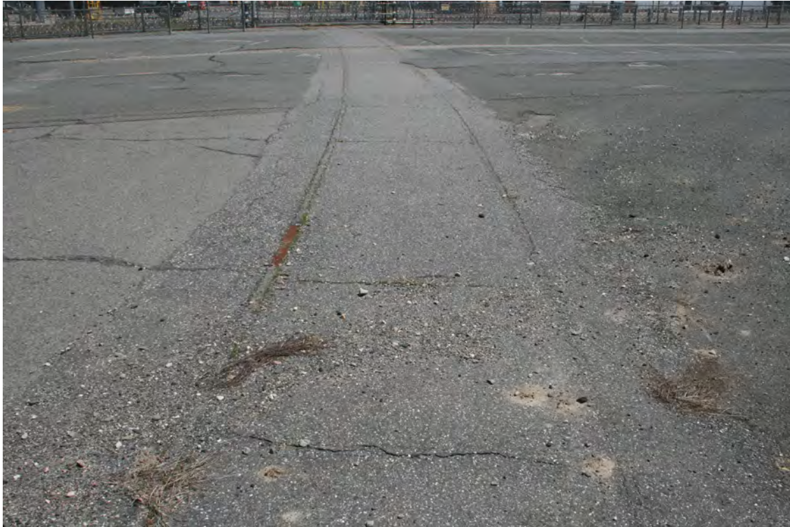
Photo courtesy of Vermont Yankee
