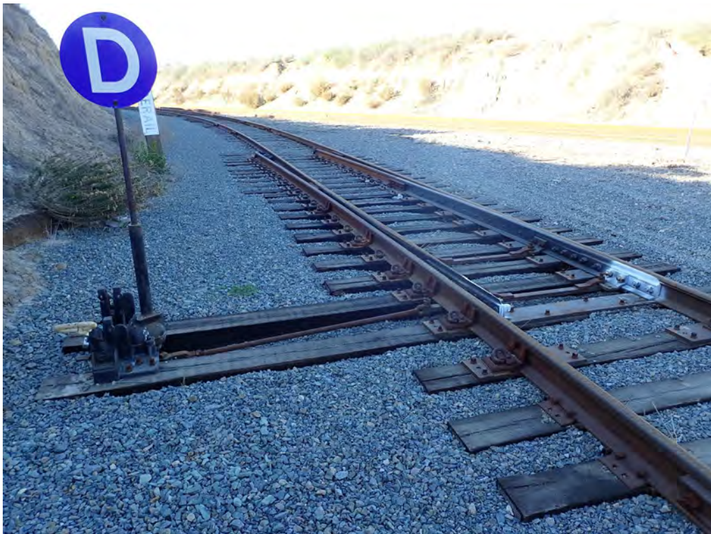
Figure 2-292. Derailer on On-site Rail Spur (2022)
