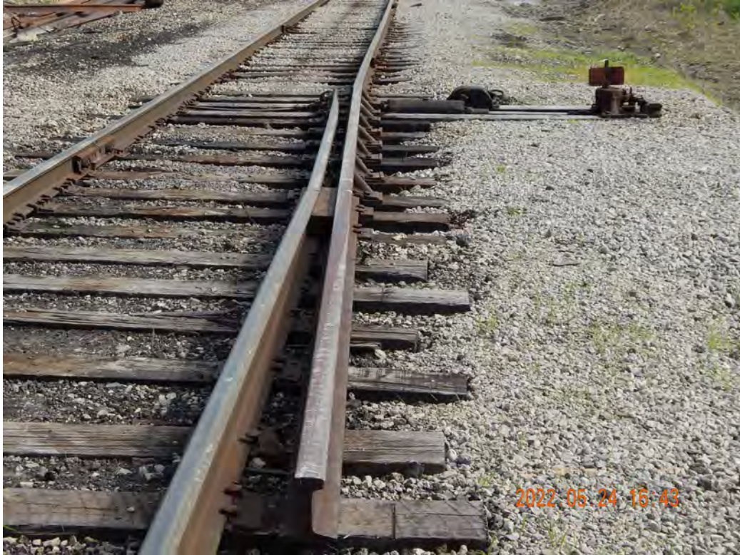
Figure 2-458. Split Derailer on Illinois Subdivision Rail Line
