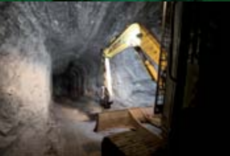
▲ The demonstration tunnel, excavated according to the design of the deposition tunnel, at final disposal depth.
