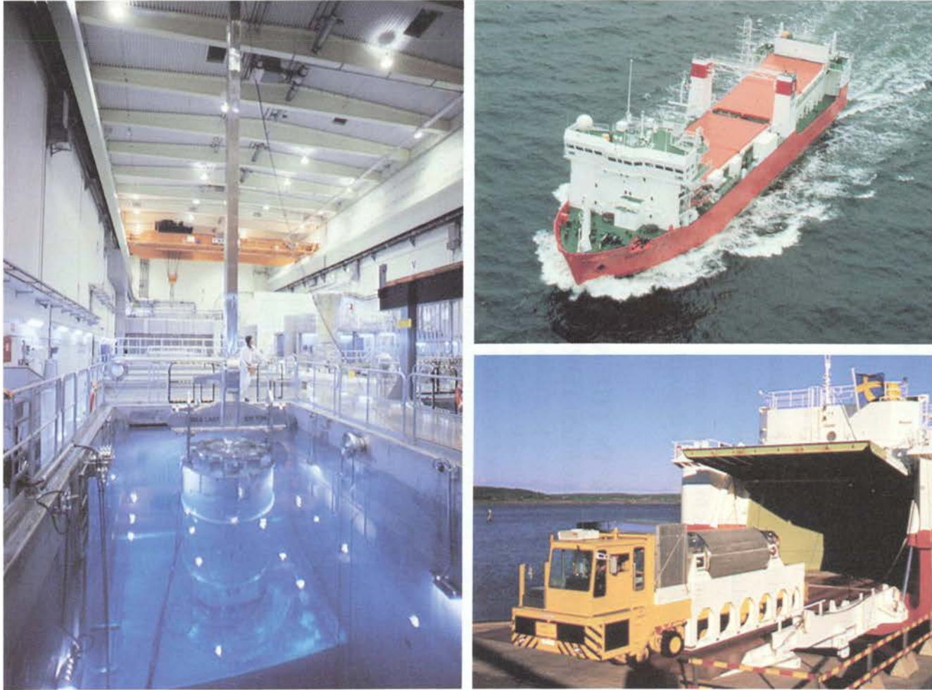
Figure 5-2 Spent nuclear fuel is stored for about 40 years in water-filled pools in the central interim storage facility for spent nuclear fuel (CLAB) at Oskarshamn. During this time, the radioactivity decays and the heat generated by the fuel is reduced by 90%, which allows for simpler handling of the fuel during encapsulation and transportation to the deep repository. However, since the level of radioactivity will still be high, the spent fuel will be transported in special containers similar to those currently used for non-encapsulated spent nuclear fuel. If the repository is located inland, a harbour terminal will be constructed for receiving and loading the fuel onto trucks or trains.
