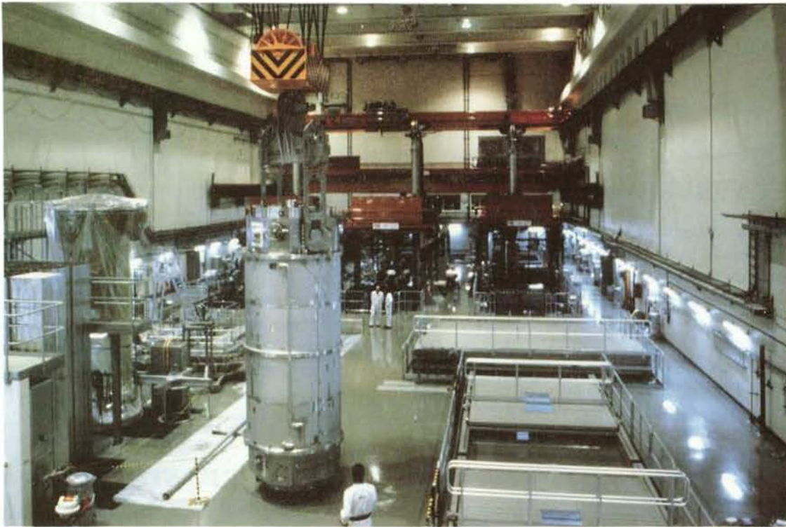
Figure 6-1. Reception building in central interim storage facility for spent nuclear fuel, CLAB.
