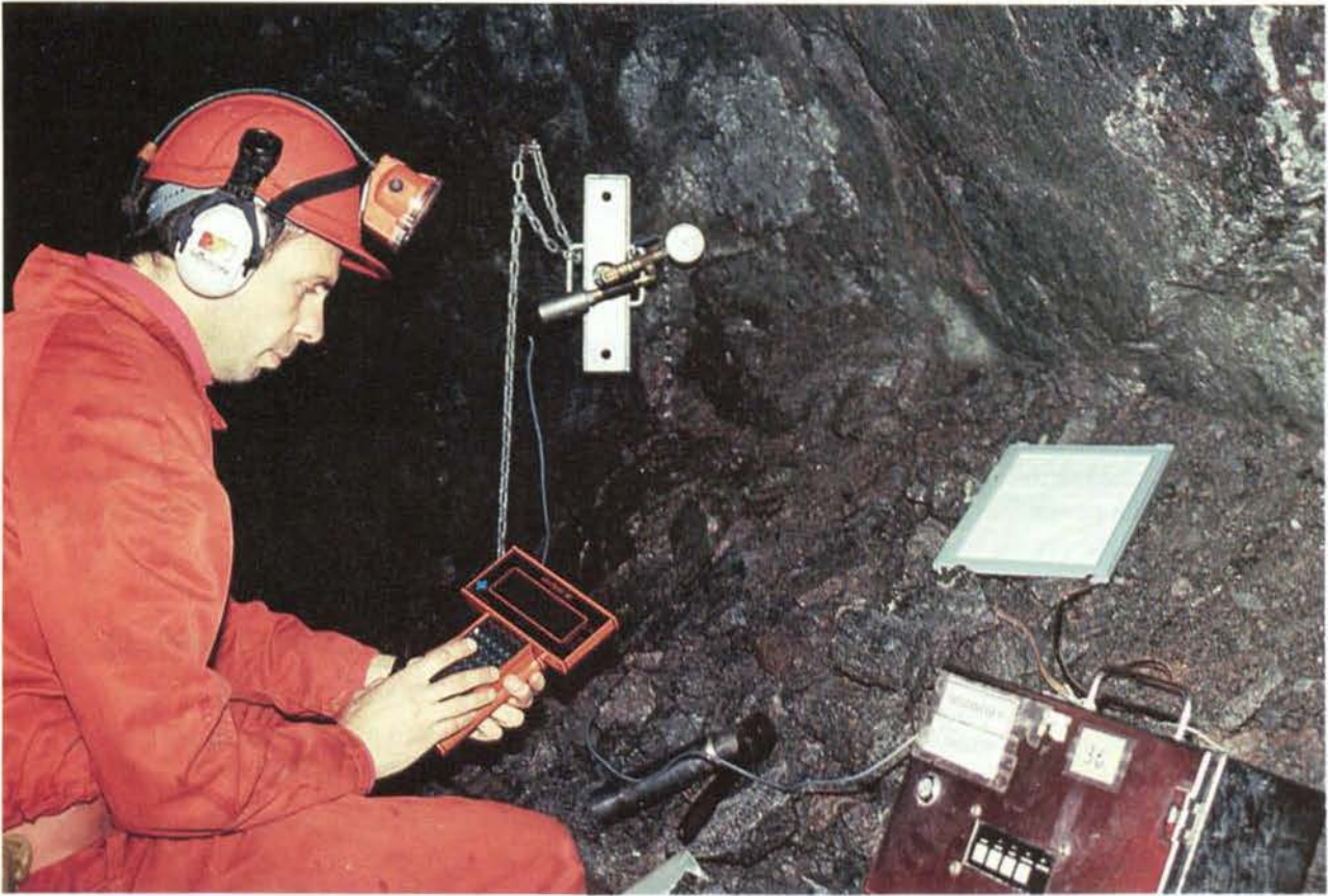
Figure 12-5. After every fourth "round", two 20 m long investigation holes are drilled in front of the tunnel. The hydraulic injection test is performed to measure water permeability (transmissivity).
