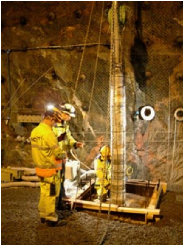
Figure 24-1. Installation of one of the parcels with 13 different materials in the “Alternative buffer materials” test in the Äspö HRL.
