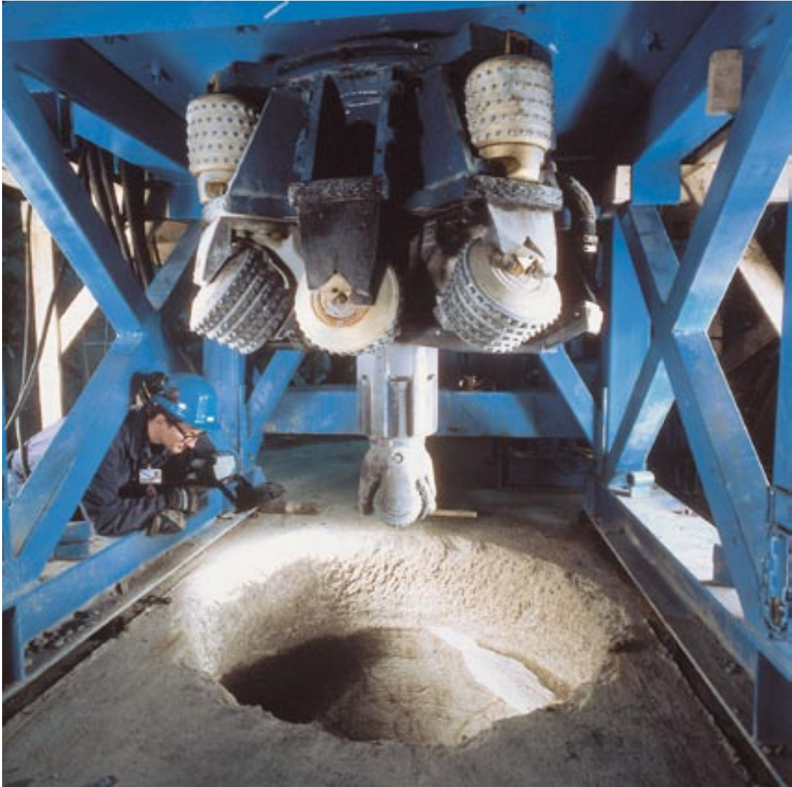
Figure 12-5. Boring of deposition holes by reverse raise boring in Olkiluoto in a joint project between SKB and Posiva.
