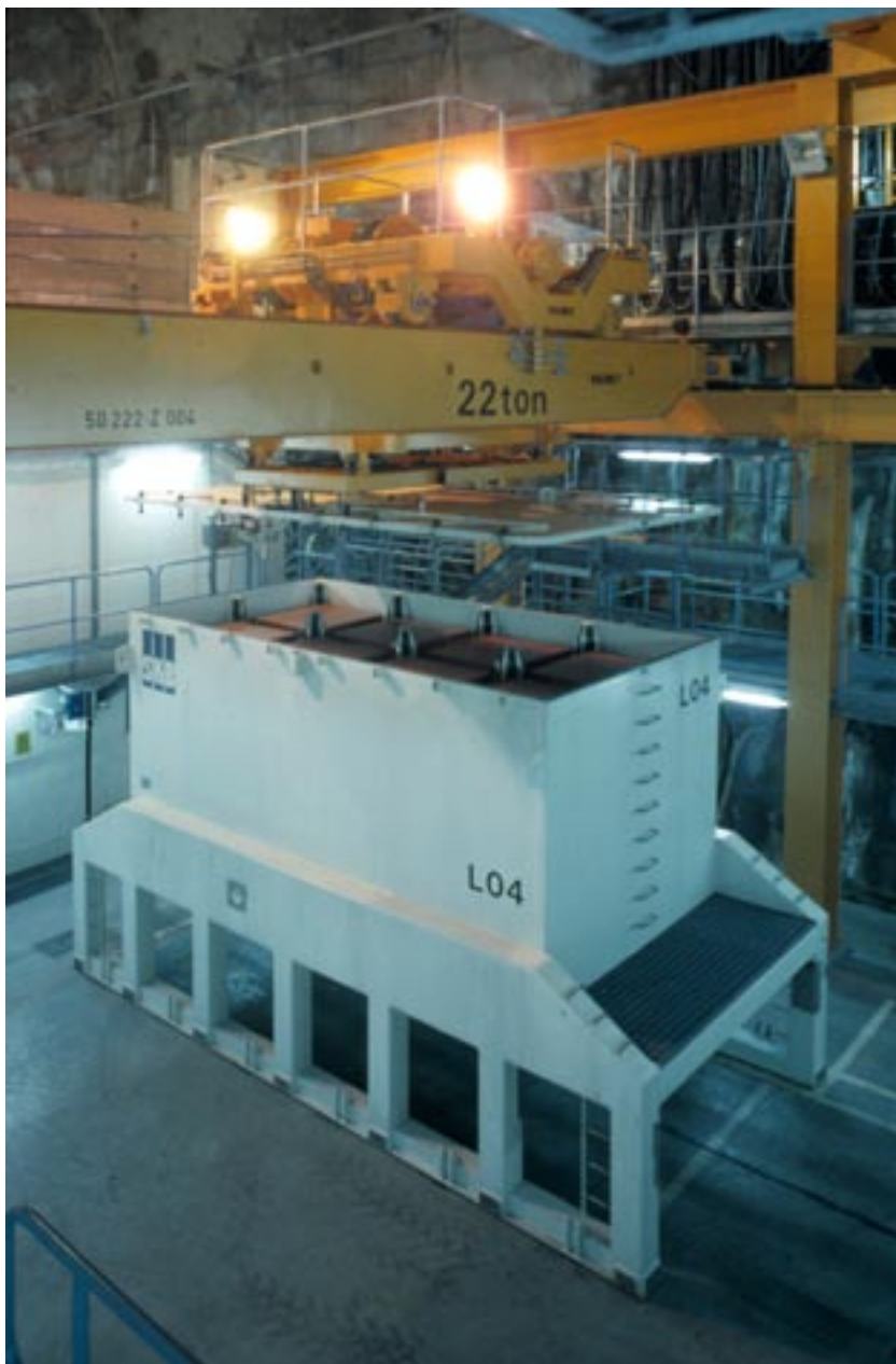
Figure 1-4. The lid on an ATB transport container for radioactive waste is lifted off.
