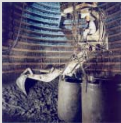
Figure 3.28 Excavation of the second shaft. Excavation of the starting chamber of the connecting gallery (top) and hydraulic arm and metal sliding ribs (bottom).
