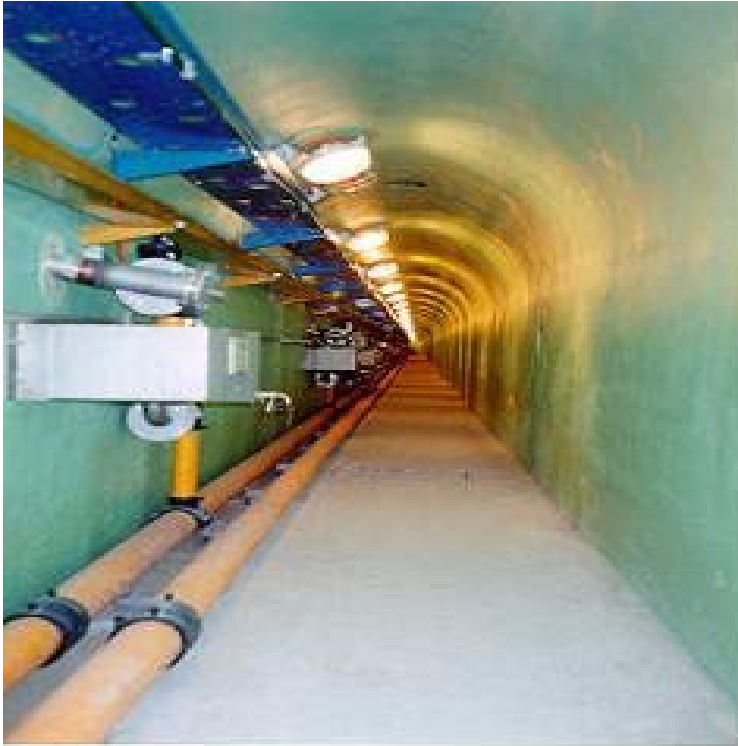
Monitoring equipment at the regional RAW repository
