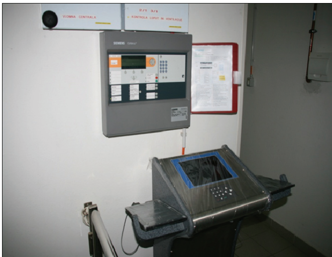
Figure 9: New independent fire alarm, located in the storage entrance hall
