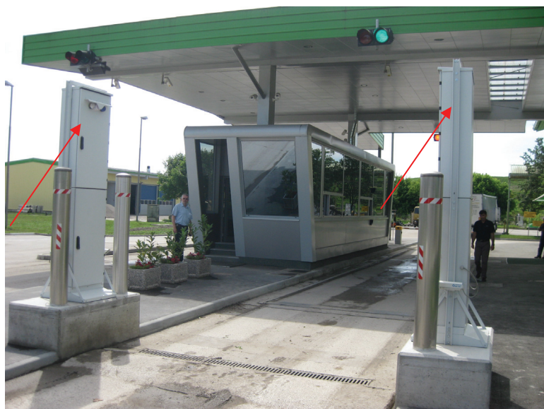
Figure 14: Portal monitors at Barje waste facility
