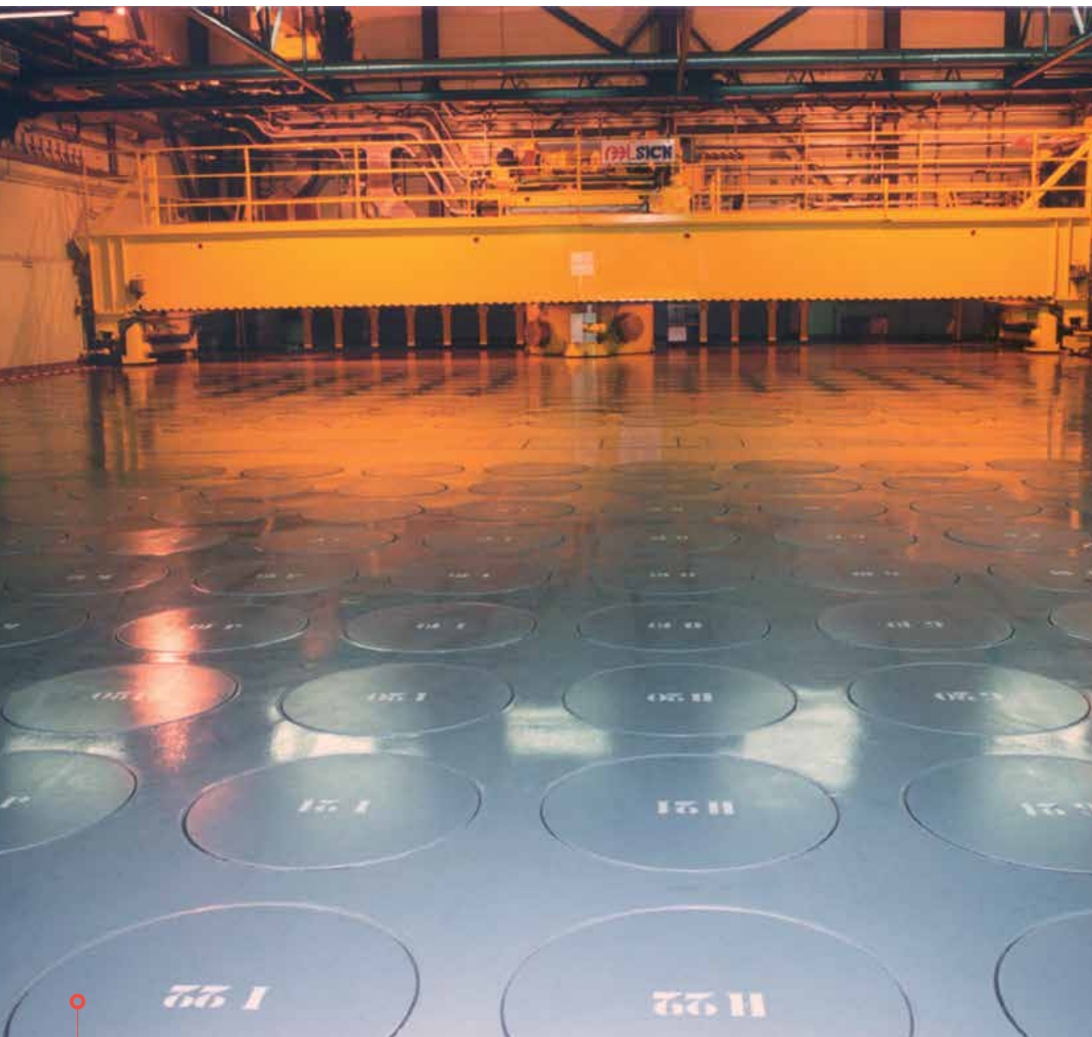
Storage hall for HLW at the Areva NC La Hague plant.
