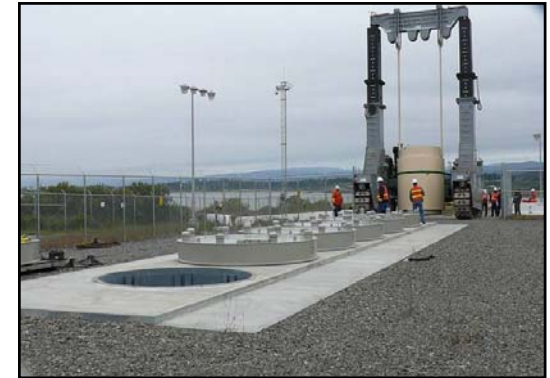
Humboldt Bay Underground Storage
