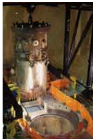
TOP: An American flag is draped across dry fuel storage container No. 7, which was loaded and moved to the nearby dry fuel storage pad. ABOVE: A special crane lifted the reactor vessel up and out of its concrete cavity, across the reactor deck and back down into its shipping container on Aug. 25, 2003.
