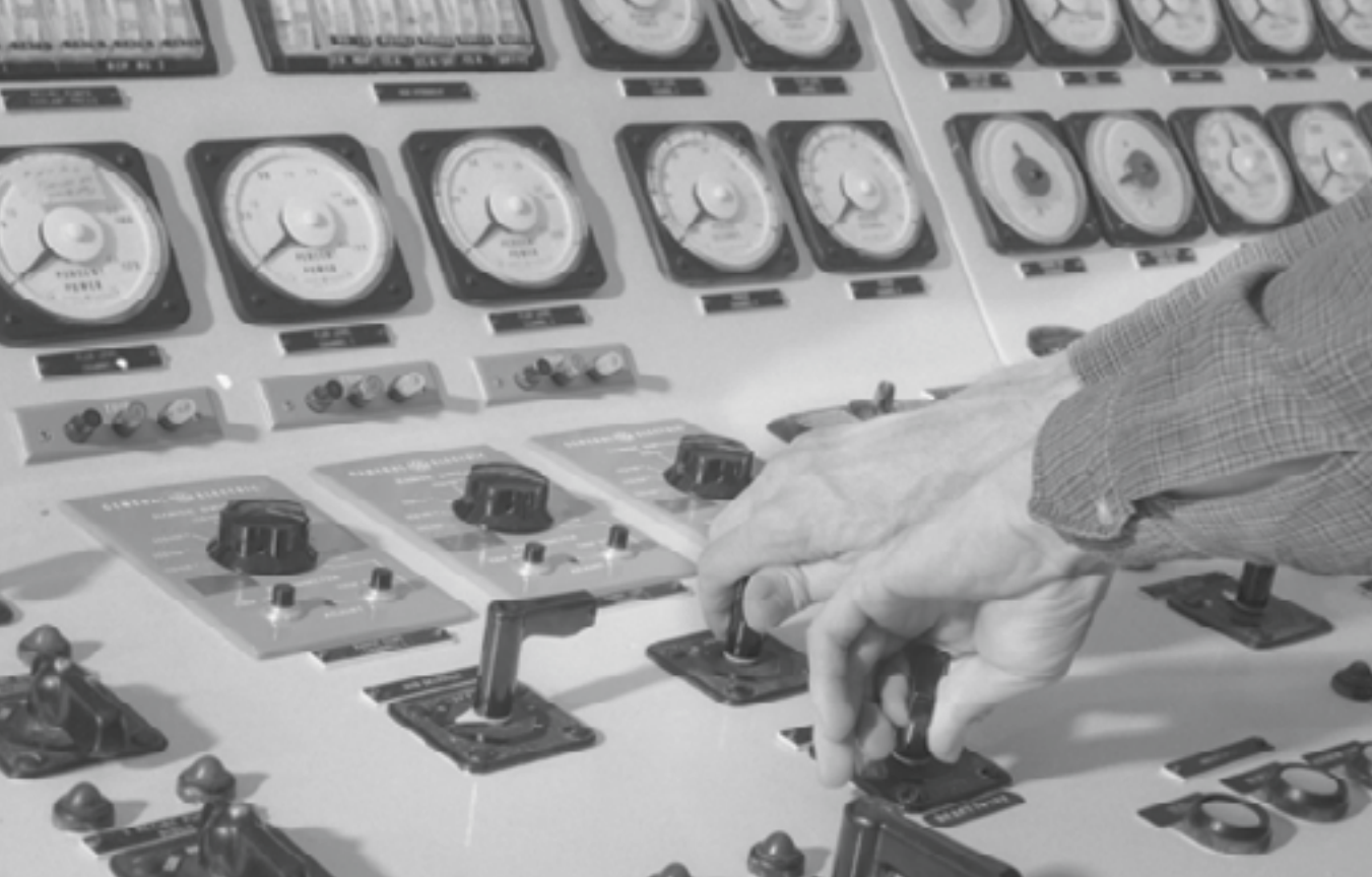
Operators manipulated control rods from inside the control room to ensure the delivery of safe and reliable electric power for northern Michigan communities and businesses for 35 years.
