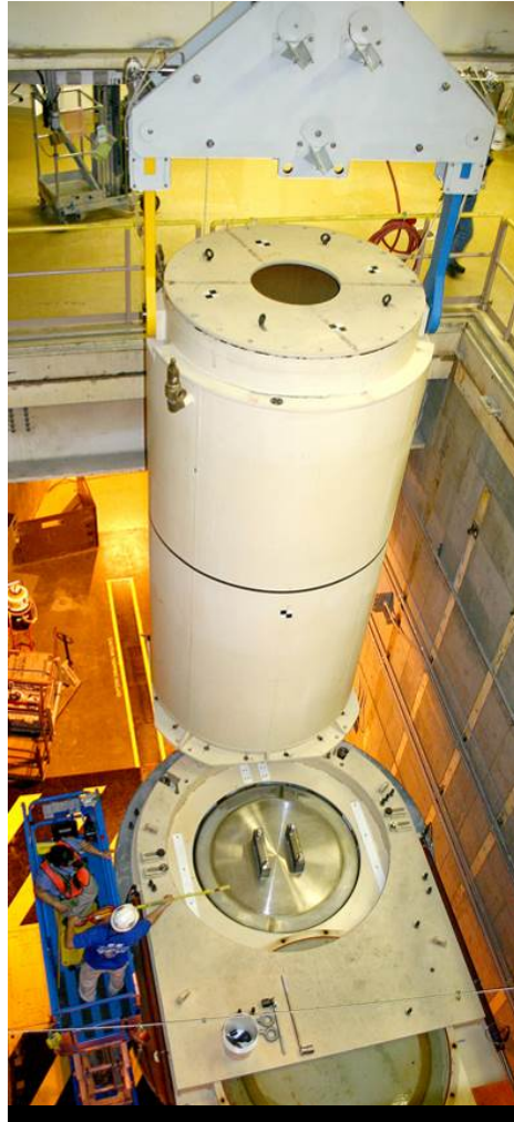
MPC Transfer Operation from HI-TRAC Transfer Cask to HI-STORM Storage Overpack
